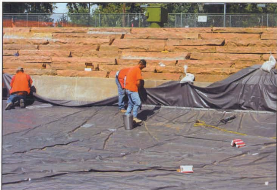
Large panels of PVC geomembrane are pulled out and battened to the concrete wall surrounding most of the perimeter of the pond.
