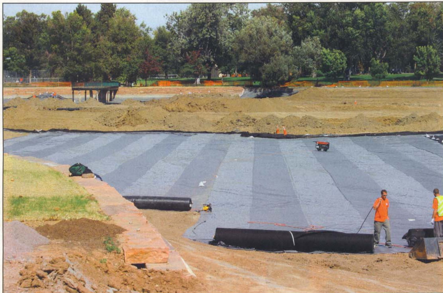
The cover soil is placed over the PVC geomembrane while work continues on the other side of the pond.
