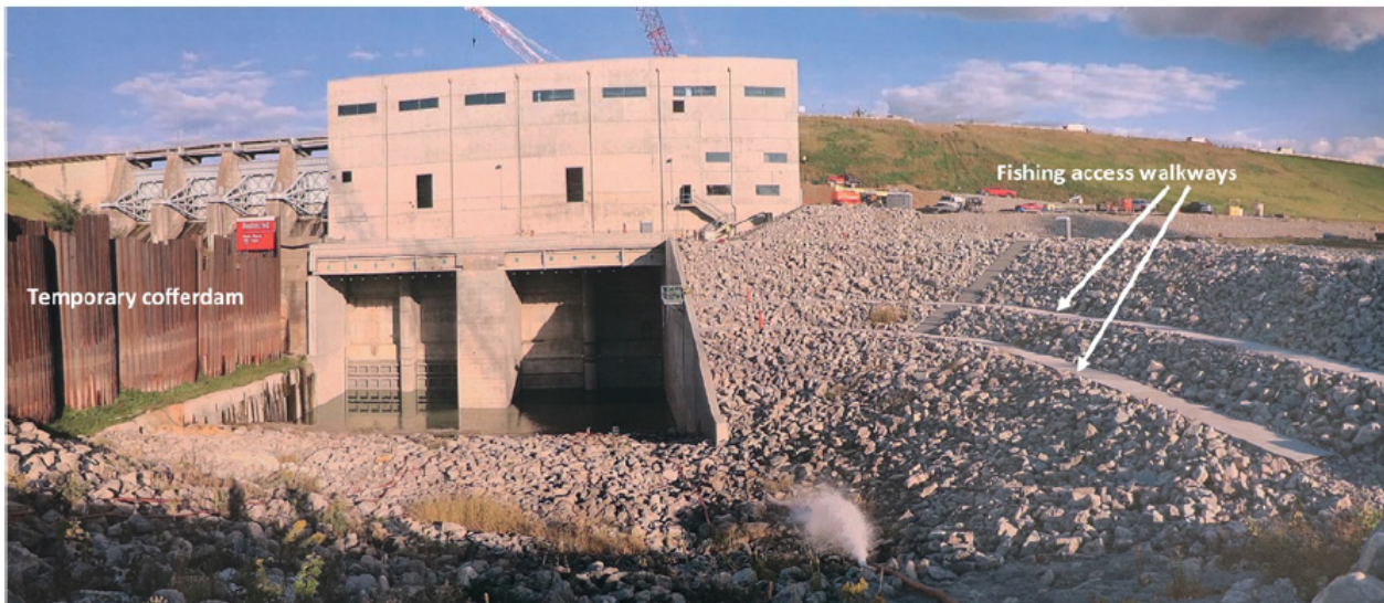
A view from the downstream side of the Red Rock Hydroelectric Project looking toward the powerhouse shows water beginning to be reintroduced into the tailrace.
