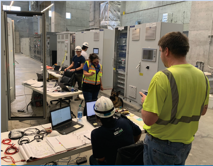
RRHP started the wet commissioning phase of Unit 2 on July 20. The commissioning process is a detailed check of every aspect of the unit's operation.
