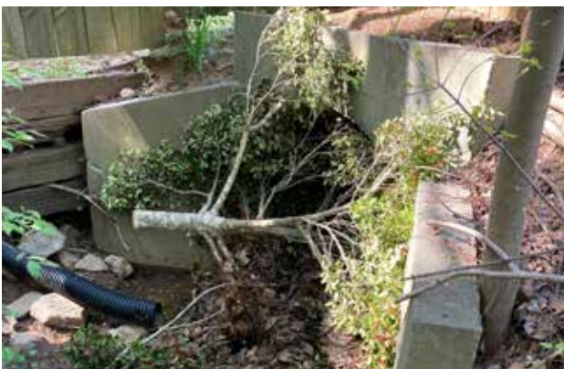
Headwall clogged with yard debris dumped by a homeowner.
