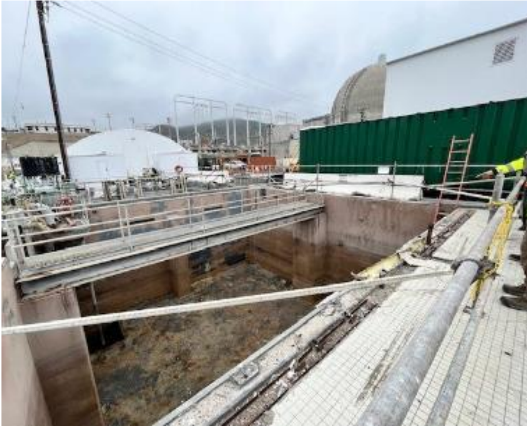
Photo 13 – Oil-Water Separator that was remediated and taken offline during the reporting period (May 28, 2024).
