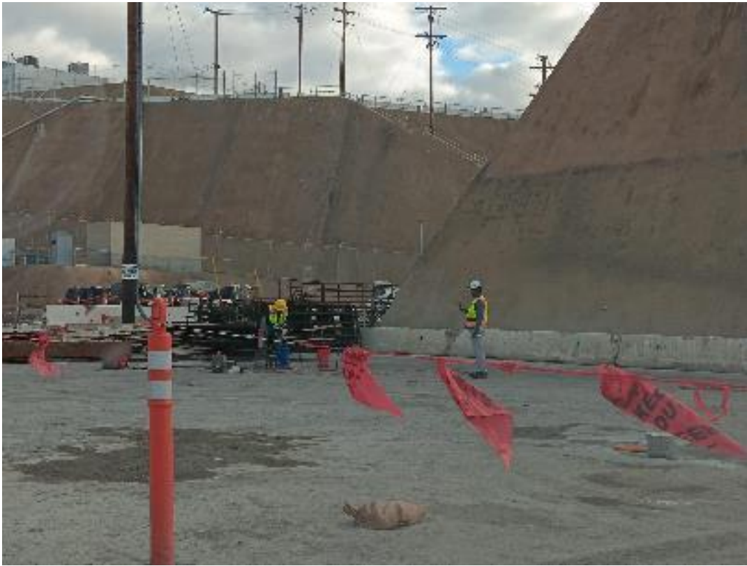
Photo 1 – Testing at an installed soil vapor probe (January 10, 2024) (photo courtesy of SCE).
