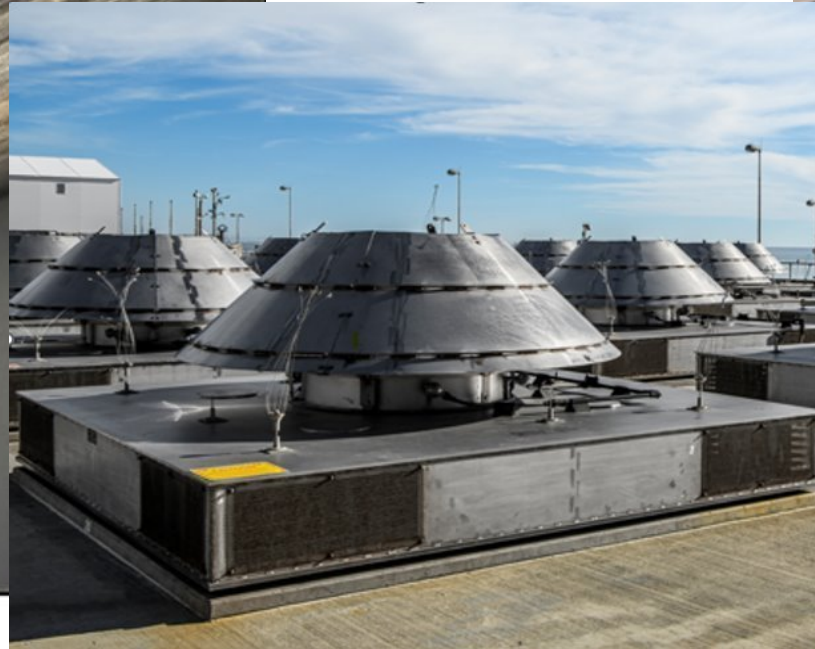
New outlet vent covers
