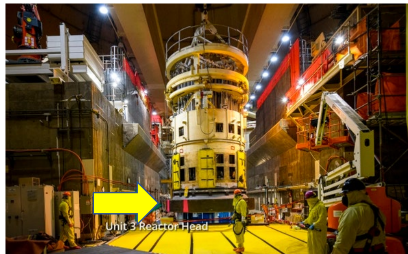
The reactor vessel head is located at the bottom of the reactor head assembly (Unit 3 pictured)
