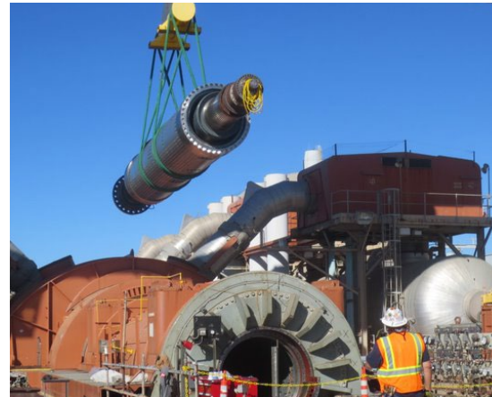
Unit 3's generator rotor has a new home. The 200-ton part was recently shipped to the Fermi nuclear power plant in Michigan.
