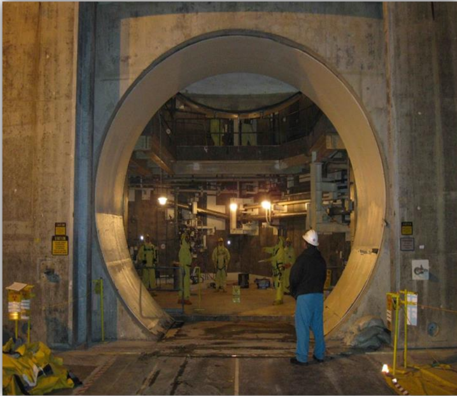
Containment Equipment Hatch Opening
