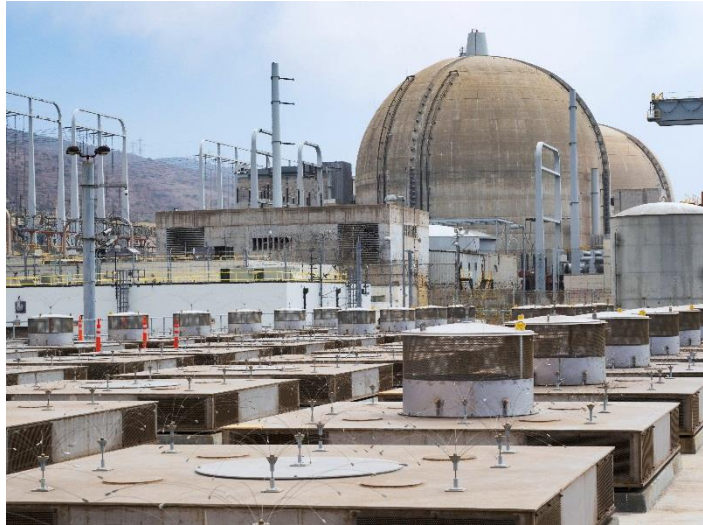
The Holtec UMAX spent fuel storage system at SONGS.
