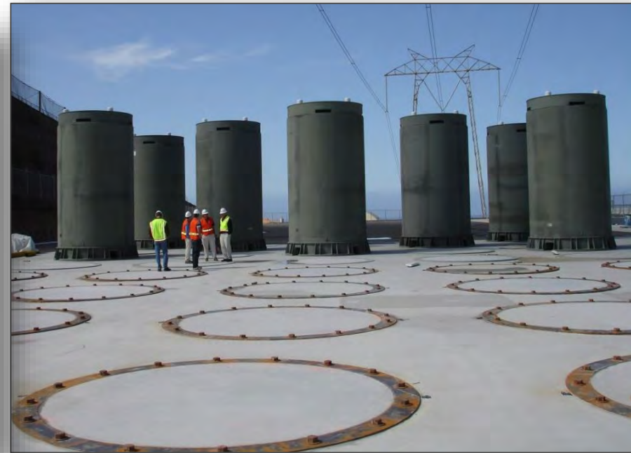
Anchored Vertical HI-STORM Systems at Diablo Canyon (2003)
