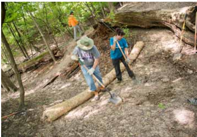
Volunteers dig a trench to support a wattle, which will in turn control soil erosion during a gully fixing workshop at Bunker Hill Forest Preserve.
