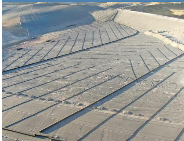
Heap Leach Pad Piping
