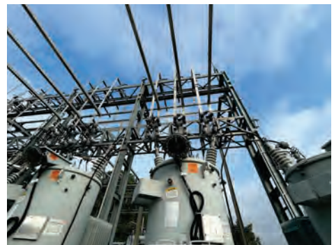
Greenwood Commissioner of Public Works One Voltage Substation
