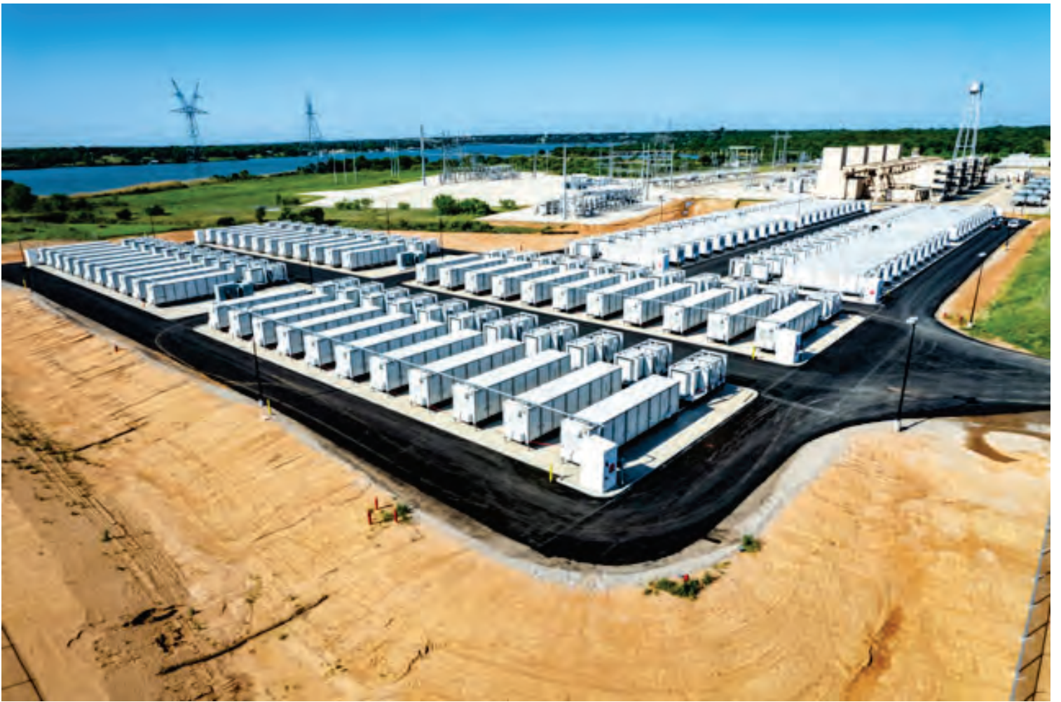
Photo: Santee Cooper rendering of possible layout for a battery storage facility.
