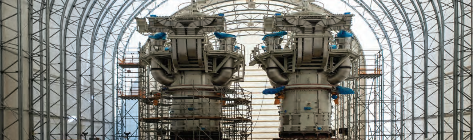
Photo: Santee Cooper, Interior of the Fairfield nuclear containment building
