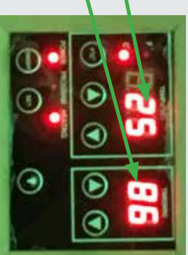
Fig1. POWER & HEATING lights illuminated to show sauna in operation
