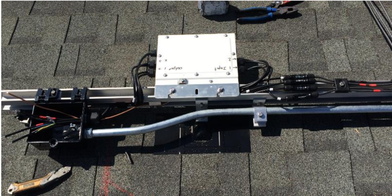
Fig 1. Typical Rapid Shutdown Device installation (RSD bonded w/ MLPE Kit, J-box and single conduit)
