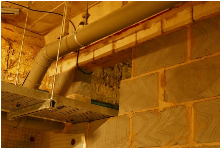
Basement Plant room, missing brickwork
