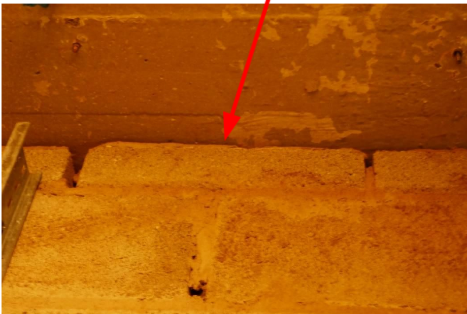
Basement area, no fire stopping where walls meet ceilings
