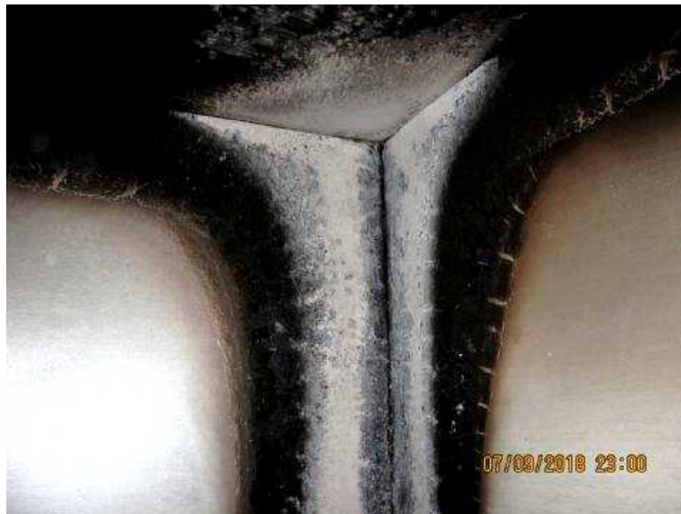
Photo No. 8 Post test photo
