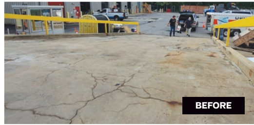
BEFORE: Slippery Ramp Surface Unsightly • Tripping Hazard
