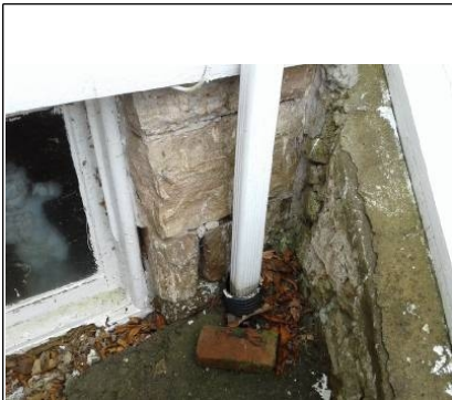
Loose missing mortar recommend tuck point repair
