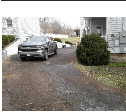
Low soil at foundation and slope towards house
