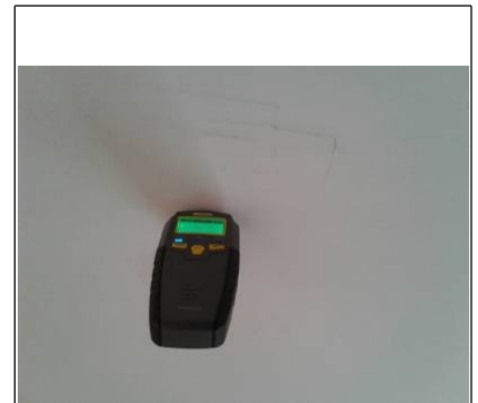
Moisture stains on ceilings
