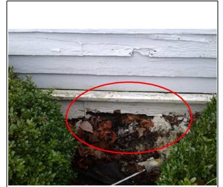
Moisture damage to sill on unit
