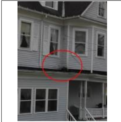
Moisture damage to wall
