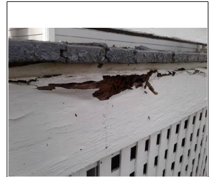
Porch wood damaged
