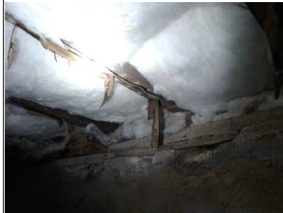
Sill not visible therefore no inspection possible to that area.
