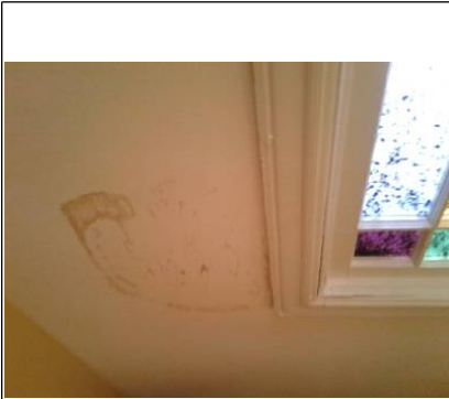
Moisture stains on ceilings
