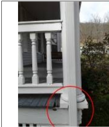
Post support damaged
