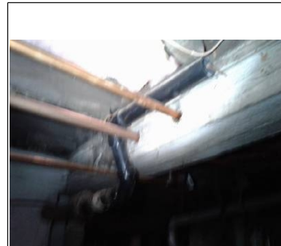
Plumbing vents in basement
