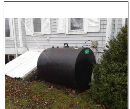
Not level. Oil line not secured
