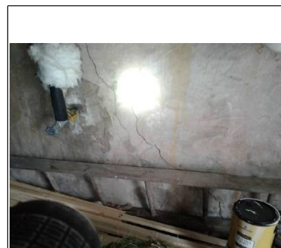
Settlement cracks and moisture stains
