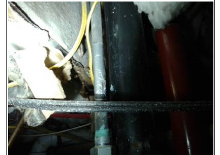
Tape on plumbing
