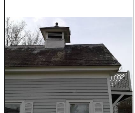
Missing shingles and moisture damage at roof and turret
