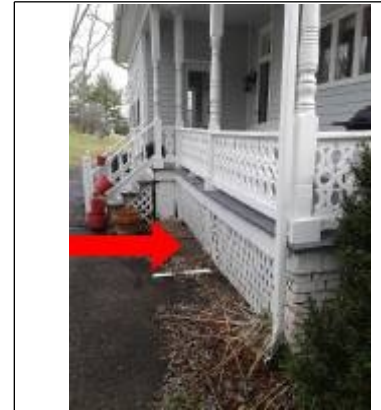
Columns and posts not plumb
