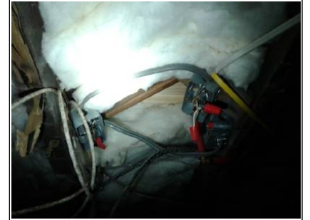
Open junction boxes
