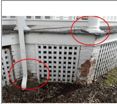
Moisture damage to wood, posts not plumb, columns leaning and bricks loose.
