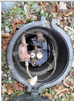
Water in access
