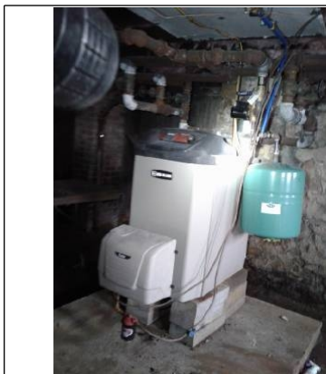
Expansion tank not supported
