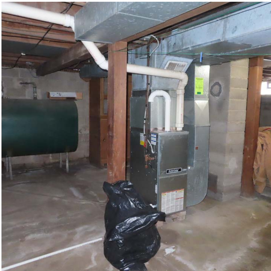
basement furnace (LP gas)
