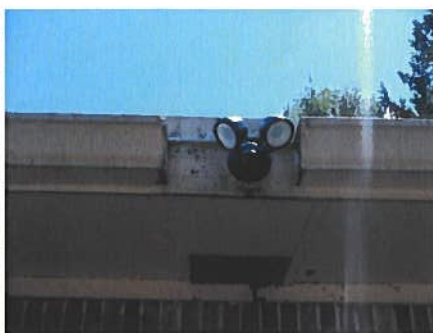
Inadequate guttering/light fixture.
