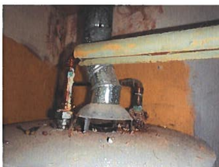
Heavily corroded water heater fitting.
