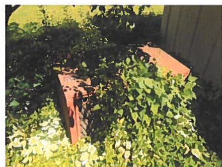
Inoperable AC condenser.
