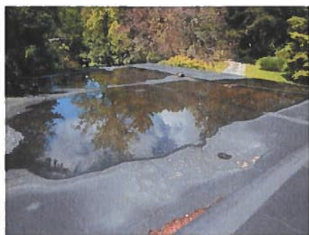
Excessive pooling water on garage.
