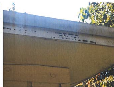
Carpenter bee intrusion at fascia.
