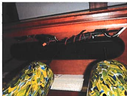
Improper wiring at kitchen light.
