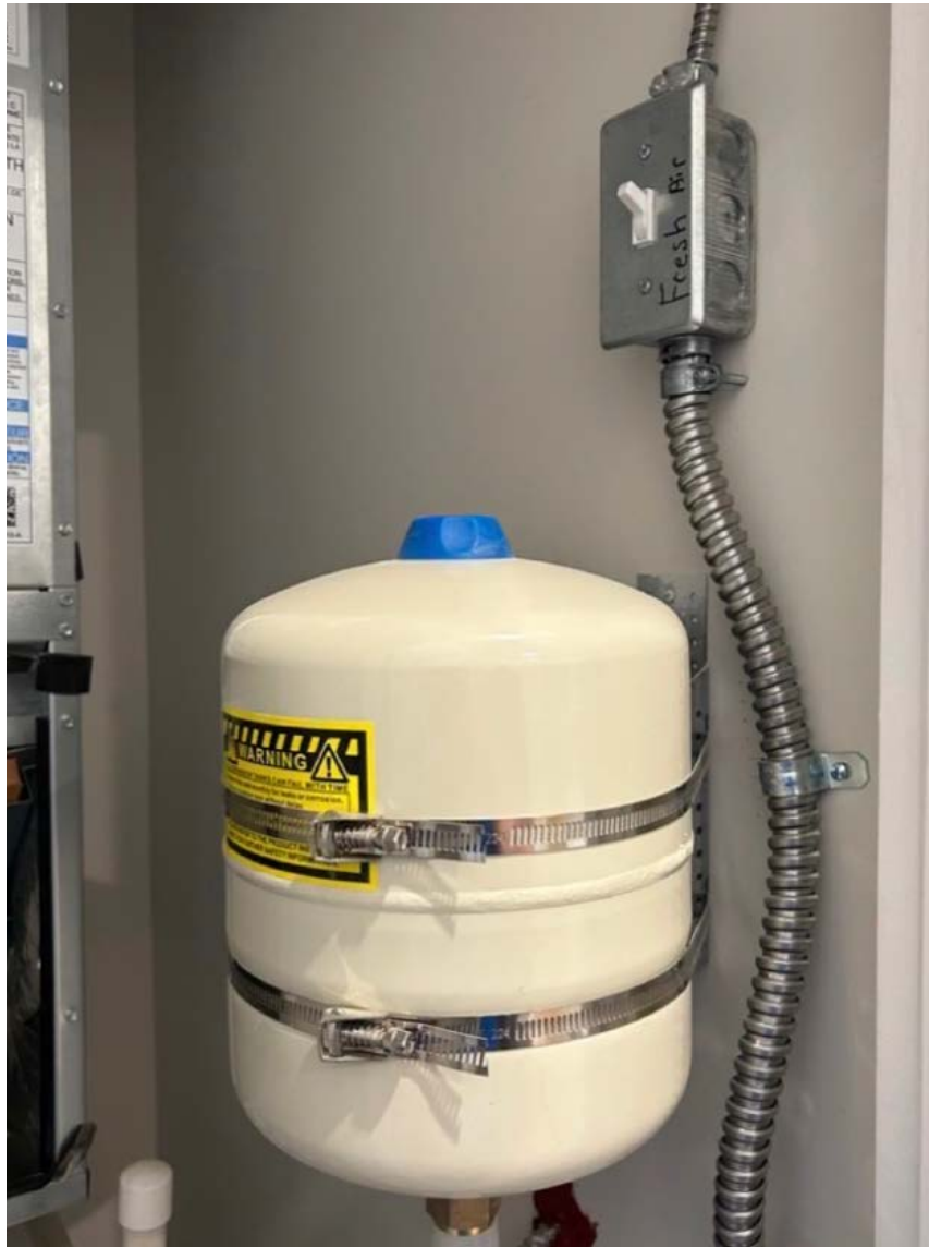
Switch for fresh air location above expansion tank
