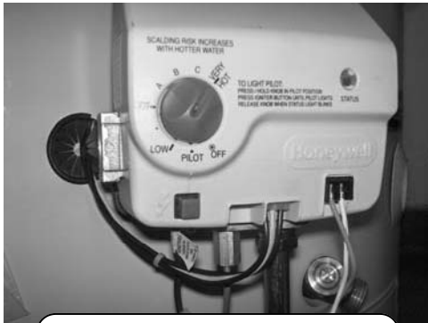
Wire harness connected to the gas control
