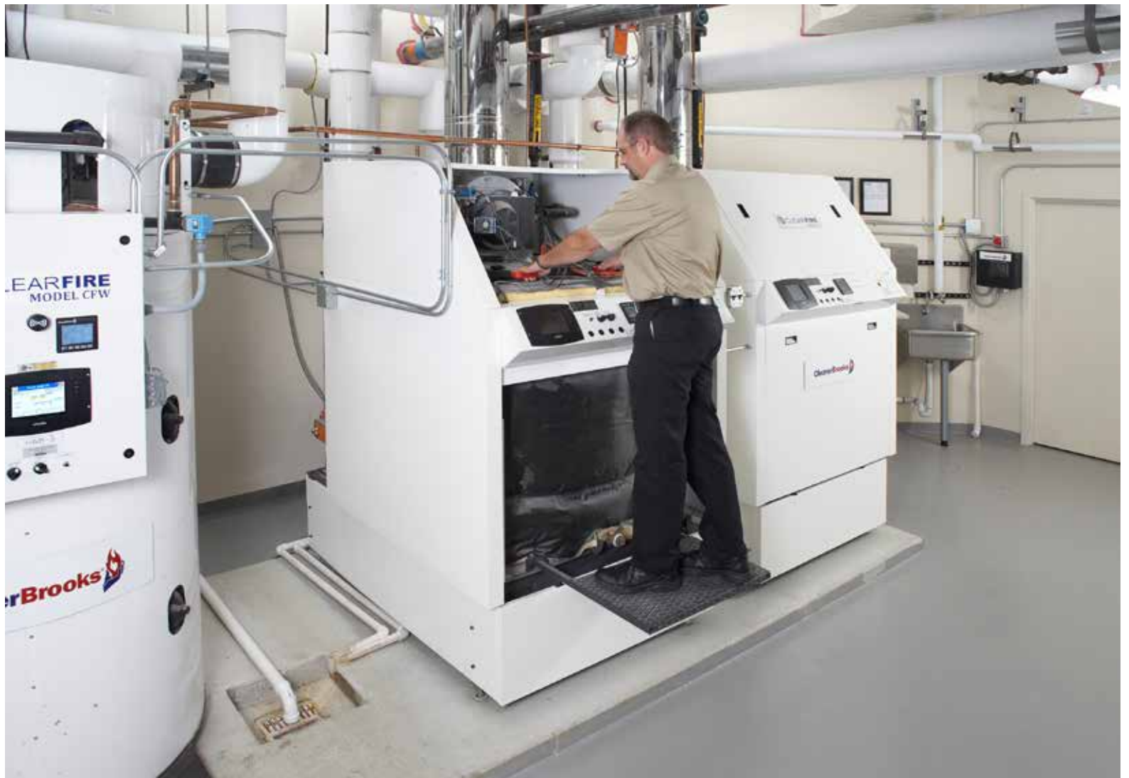
OPTIMIZED BOILERS: Often the simplest way to optimize energy efficiency in condensing boilers is to lower the return water temperature to the point the system is operating in condensing mode. PHOTO COURTESY OF CLEAVER BROOKS INC.
