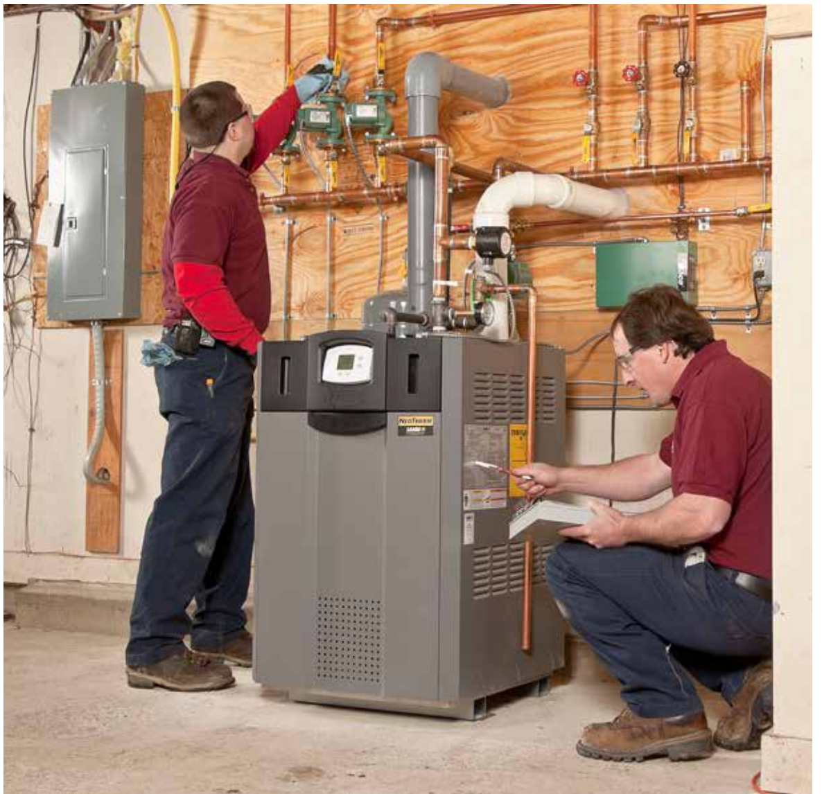
BOILER INSTALL: Technicians from Rymes Propane & Oil, Concord, New Hampshire, complete commissioning of a light commercial Laars NeoTherm boiler installation at Shoals Marine Laboratory on Appledore Island, New Hampshire.
