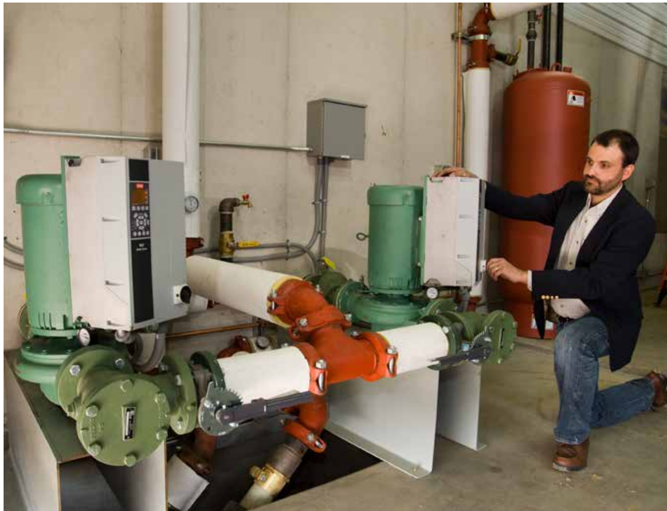
CONSTANT CONDITIONS: Self-sensing pumps can help improve efficiency by responding to the demands of the system and delivering a constant temperature differential across the boiler(s) at variable flows. PHOTO COURTESY OF TACO COMFORT SOLUTIONS
