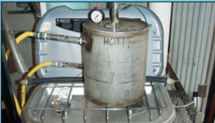
Part of VRI's methane refinery.
