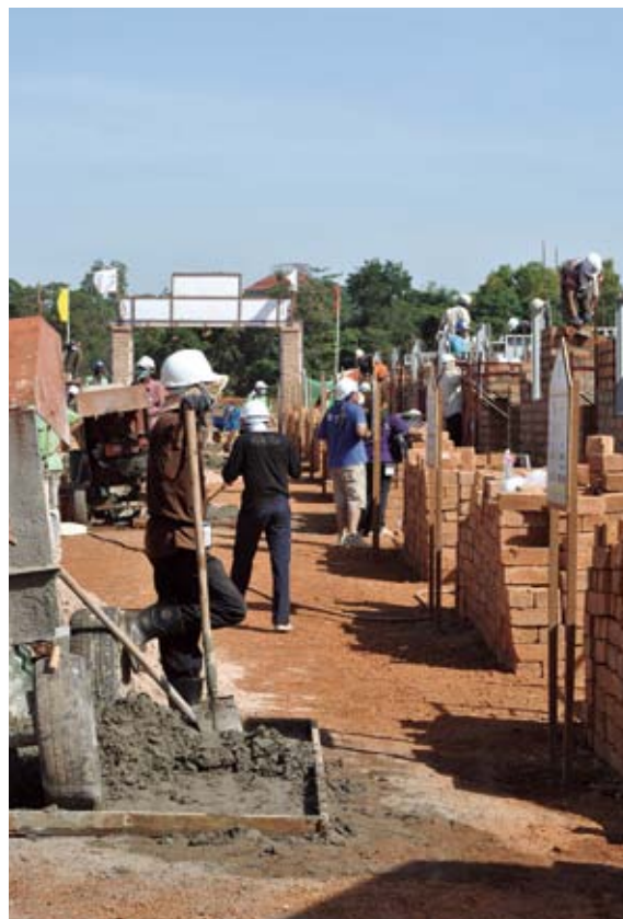
International volunteers with Habitat for Humanity construct a row of houses in the ancient capital city of Oudong, in Cambodia's central region.
