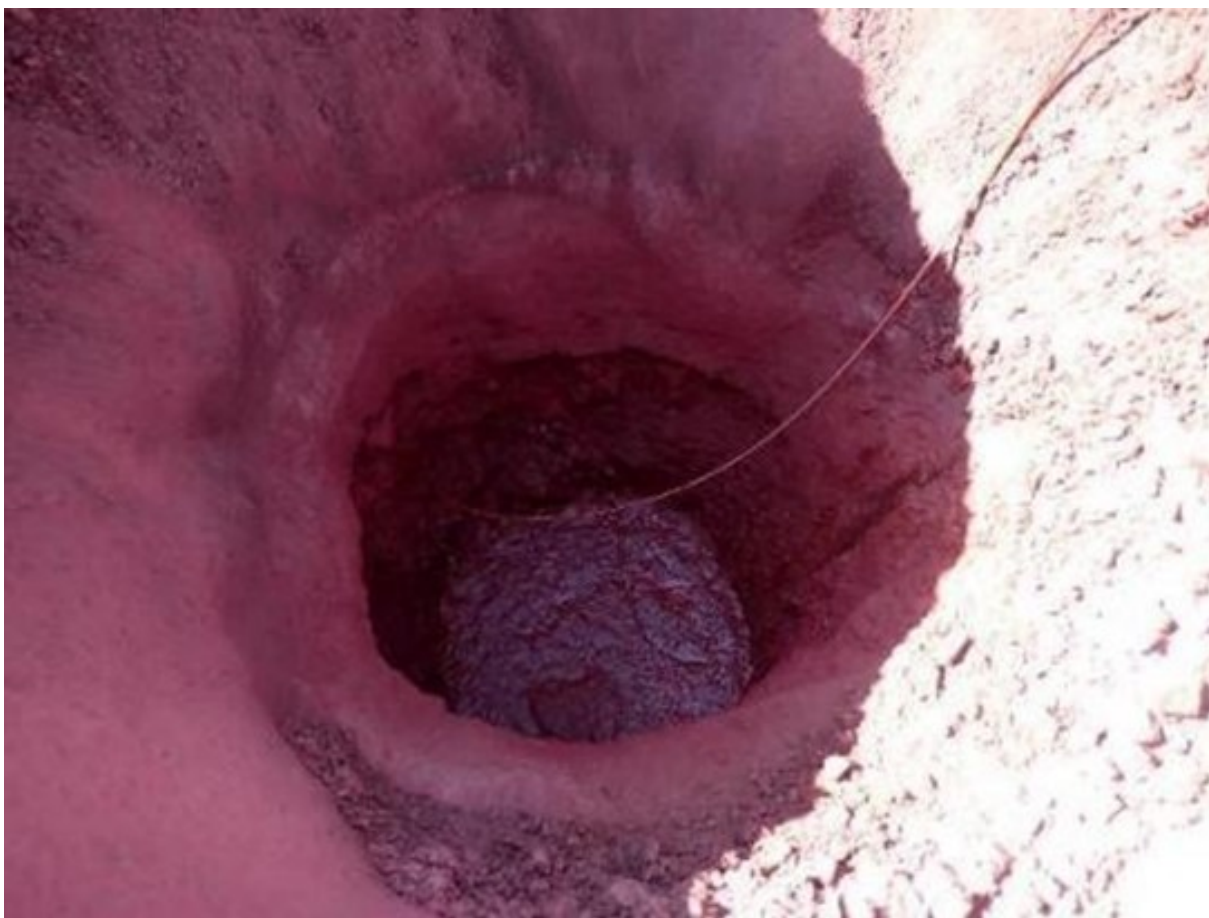
Figure 1 Decomposed straight gassed bulk emulsion at the collar of the blast hole.
