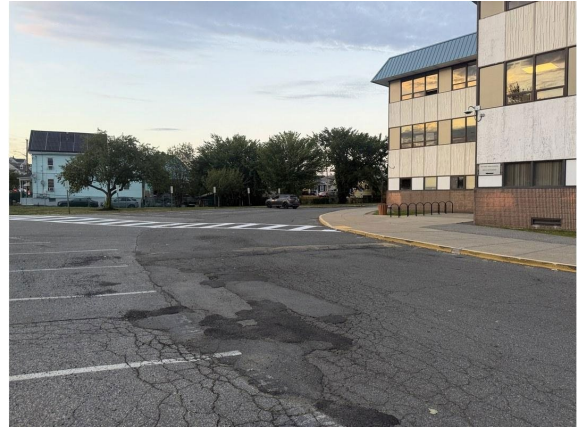
Revere High School view showing the worn roadway surface and existing speed bump area near a marked pedestrian crossing.
