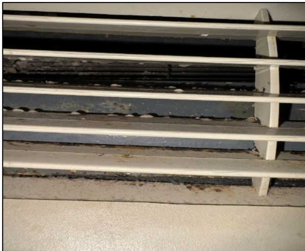
Figure 1: Growth inside heating/cooling unit at the Sleep Inn
