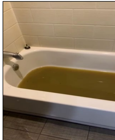
Figure 2: Tub drain backing up
