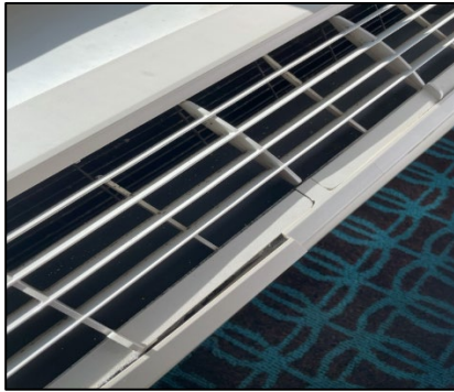
Figure 10: A/C unit in Room 257
