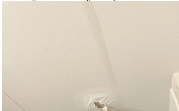
Figure 8: Water damage Holiday Inn Room 512
