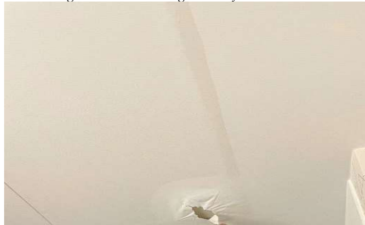
Figure 8: Water damage Holiday Inn Room 512
