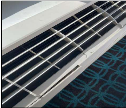
Figure 10: A/C unit in Room 257
