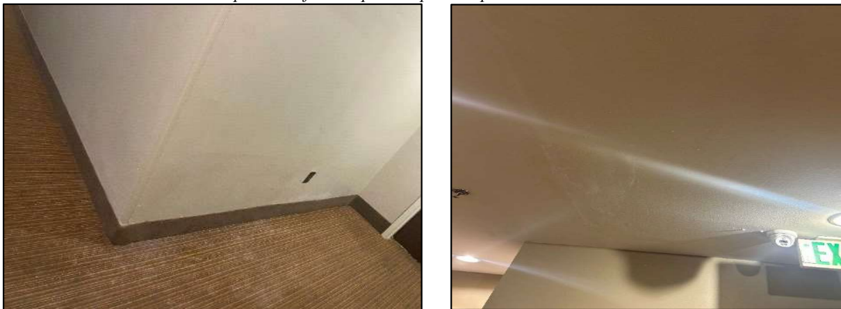
Figure 9: Photos that MOHS Director provided for Sleep Inn repairs September 2025
