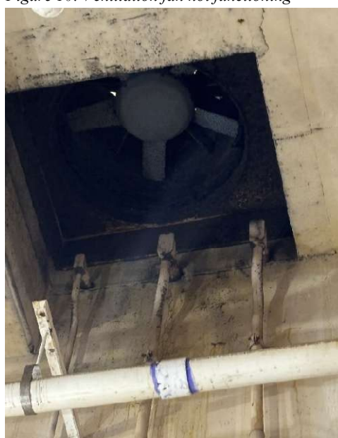
Figure 10: Ventilation fan not functioning
