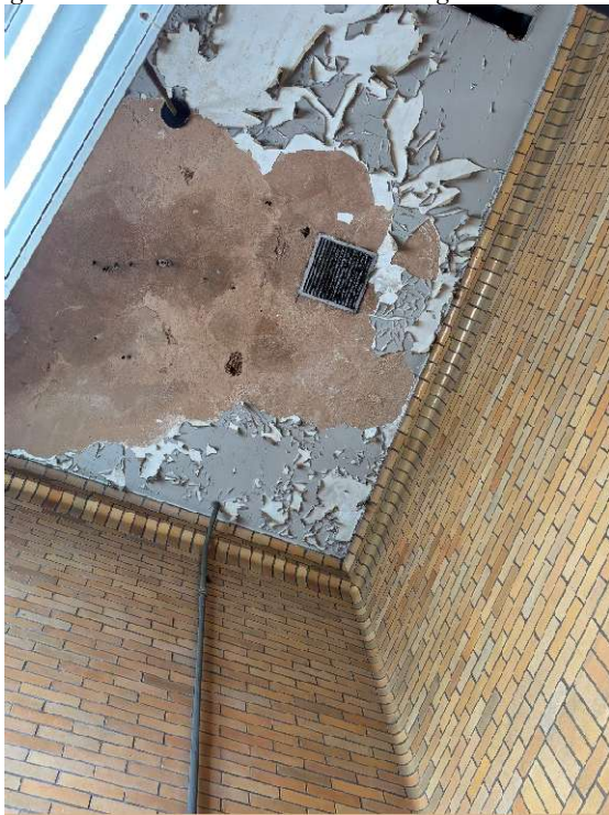
Figures 19&20: Bathroom area and ceiling
