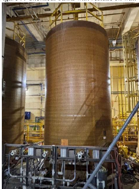
Figure 9: Chemical Tanks with residue on wall
