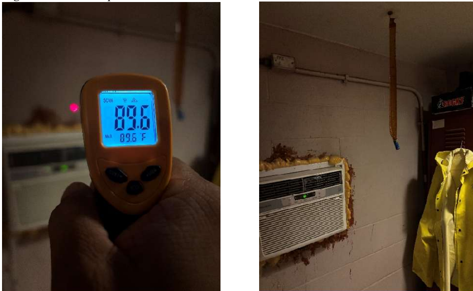
Figures 3 and 4: Temperature and air-conditioner in men's locker room area
