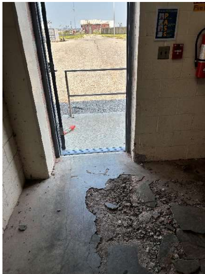
Figures 1 and 2: Flooring at doorway
