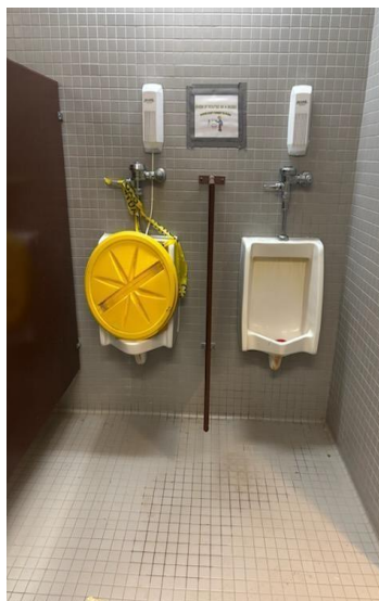
Figure 8. Men's Room Urinals
