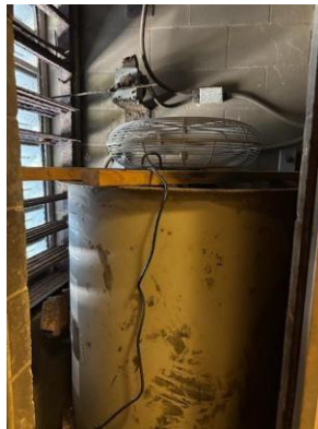
Figure 9. Temporary fan for RSPS exhaust
