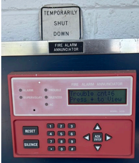
Figure 14: Trouble codes on fire alarm system
