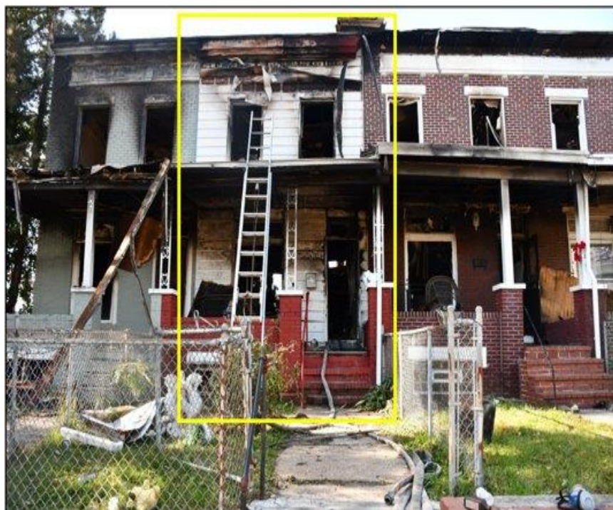
(Photo 14: Exterior of Side Alpha of 5210 Linden Heights as outlined in yellow.)
