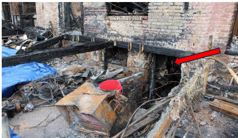
(Photo 5: 5210 Linden Heights deck joists and ledger board from previous deck construction that served as a base upon which the addition was built.
