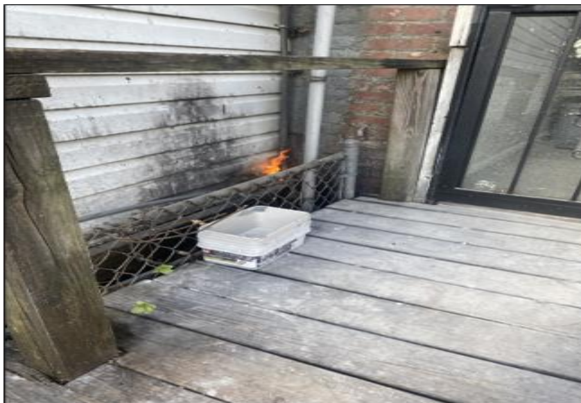
(Photo 7: Fire venting from the exterior wall of the first-floor rear addition of 5210 Linden Heights Avenue, adjacent to 5208 Linden Heights Avenue where contractor was working.)
