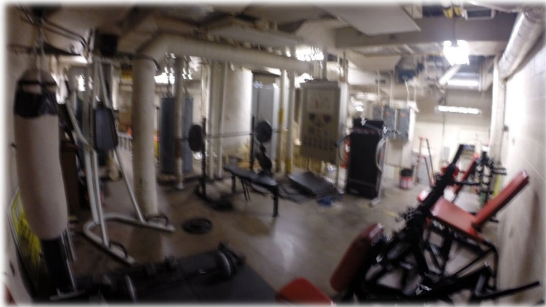
Weight room in basement with utilities
