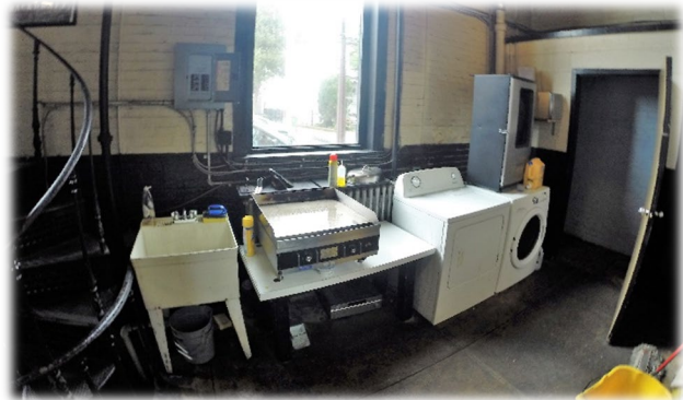
Laundry tub, cooking griddle, & laundry in bays
