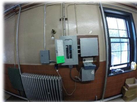
Electrical panel in bay
