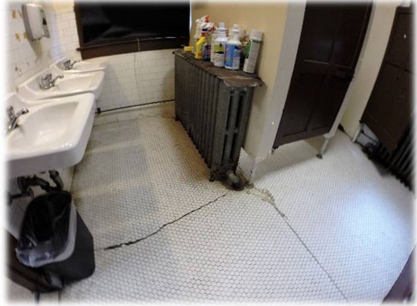
Cracks in floor and wall
