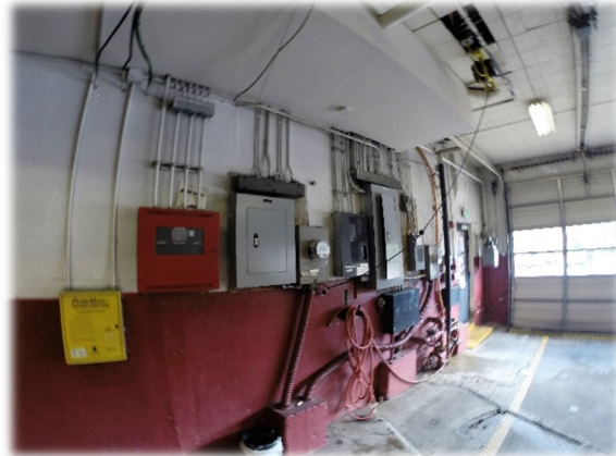
Main electrical service
