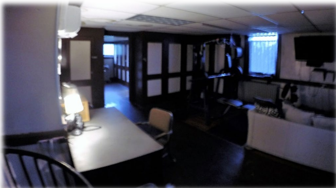
2 nd floor stair landing is open
