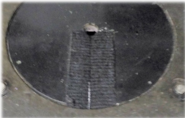
Abandoned pole hole is secured but not sealed
