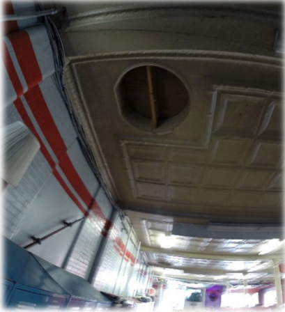
Abandoned pole hole
