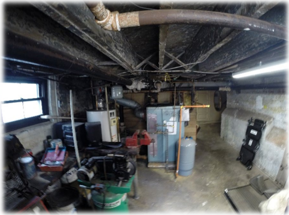
Utilities and storage in basement
