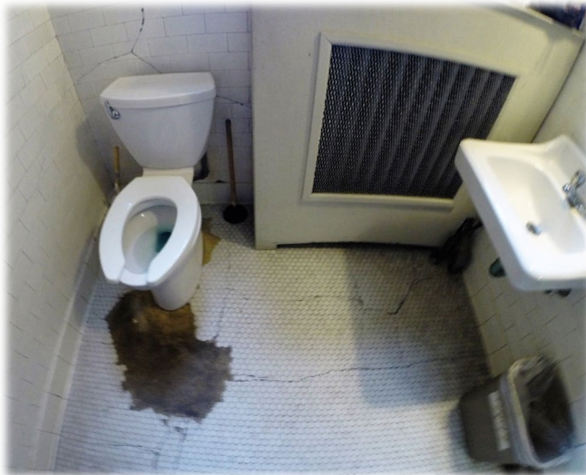
Captain's private restroom – floor and wall cracks
