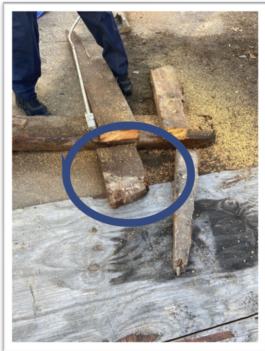
Figure 15 Example of joist pocket from 205 S. Stricker Street (BCFD Member)
