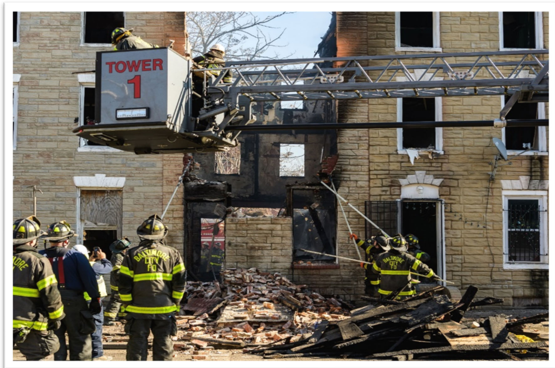
Figure 72 Members work on removing bricks from first floor of Side Alpha (Stanley Jaworski)
