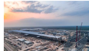
Sinton, TX 2 Greenfield EAF Steel Mill • 3.0M Tons • 1 Galvanizing Line • 1 Paint Line
