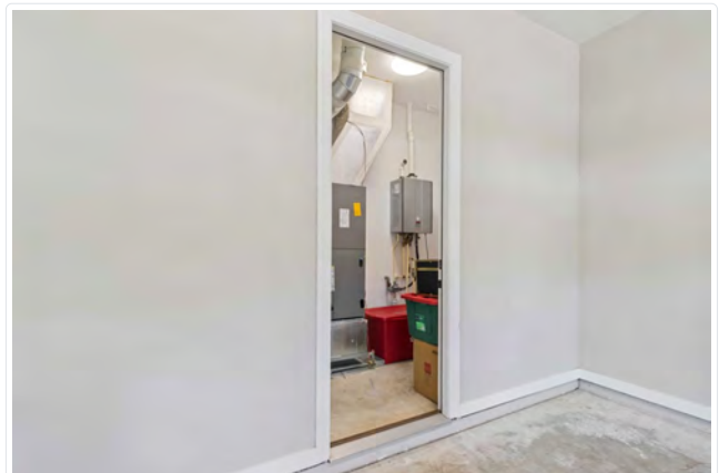
Mechanical room in main home 3-car garage
