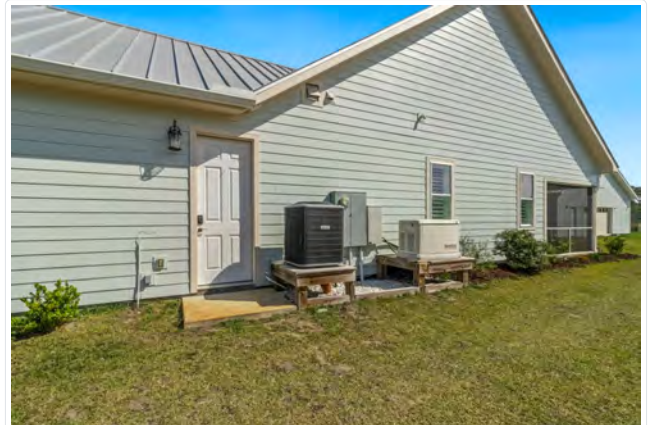
Door into Mechanical Room of garage
