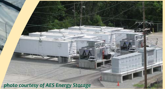
photo courtesy of AES Energy Storage
