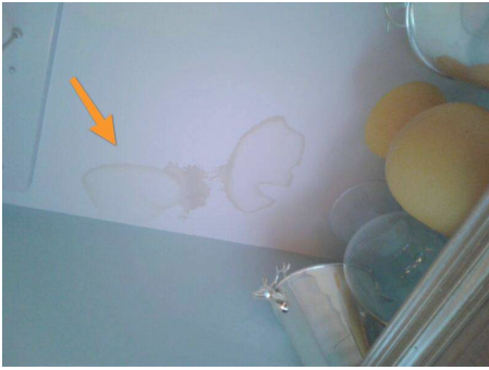
1st floor laundry
