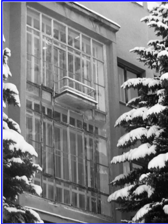
Figure 33 Ginzburg, Ordžonikidze sanatorium, west façade of east wing with glass curtain wall and floating balcony
