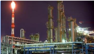
Indonesia – Installation and pre-commissioning of Nippon Shukobai acrylic plant gas turbine generators
