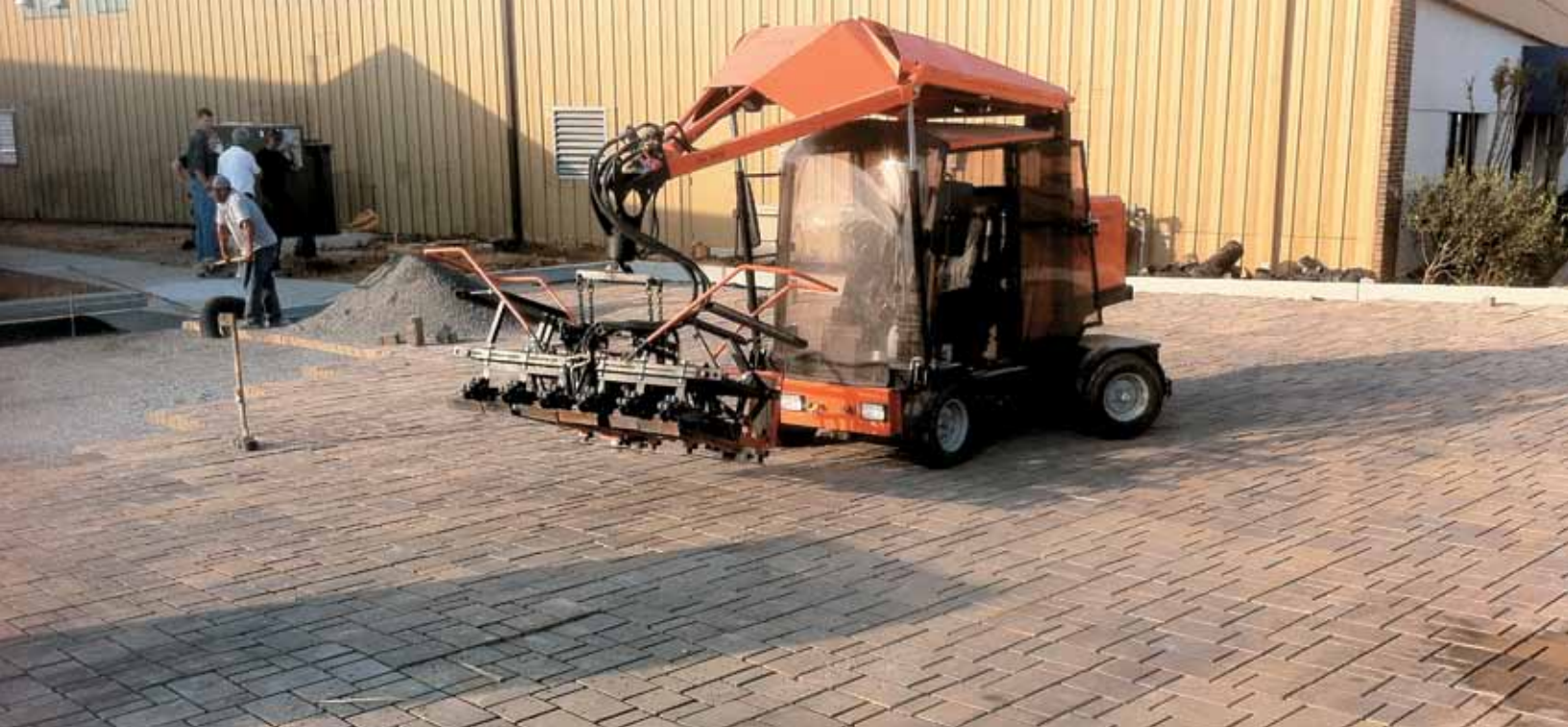
Mechanical installation of commercial parking lot. Location: Marietta, Georgia
