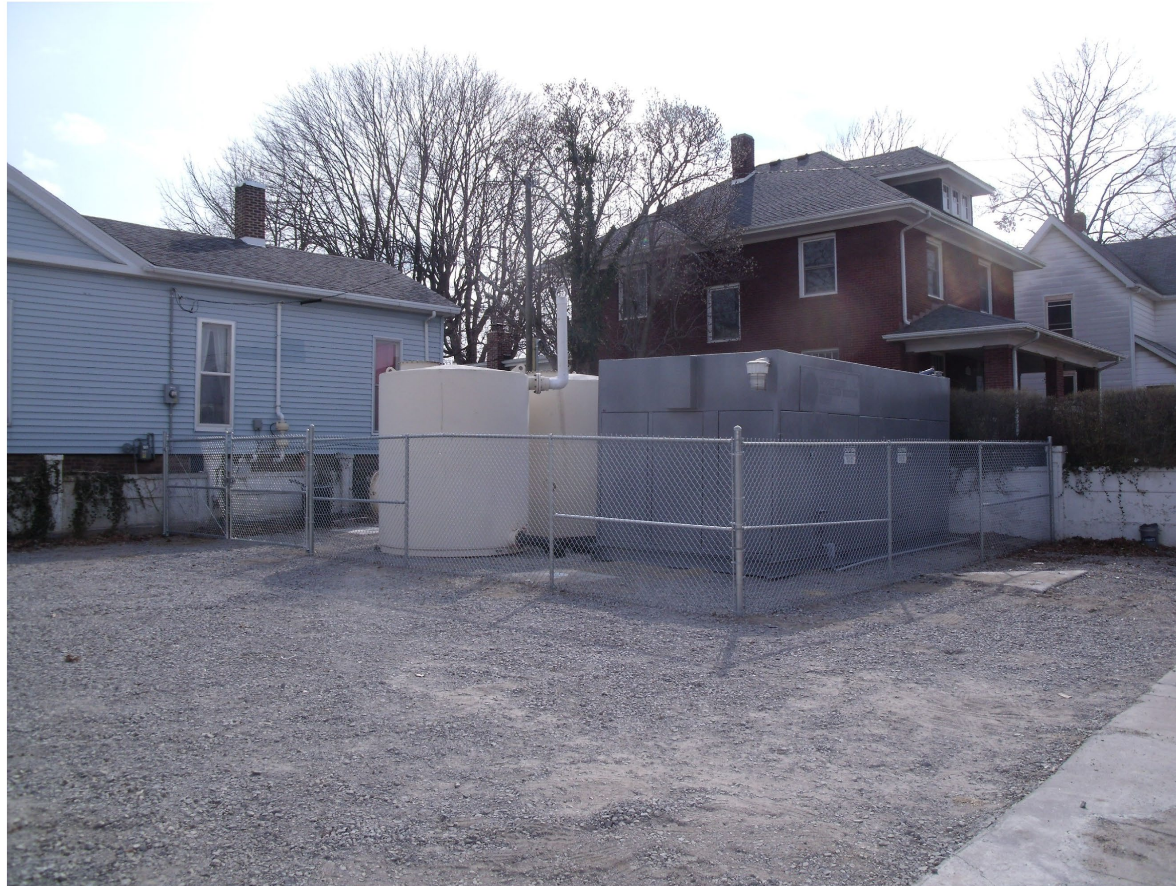
Figure 4 _ SVE System: A 1000 CFM PD blower enclosed in a Cargo container and two 8000 lbs (filled 5000) Granular Activated Carbon (GAC) Vessels
