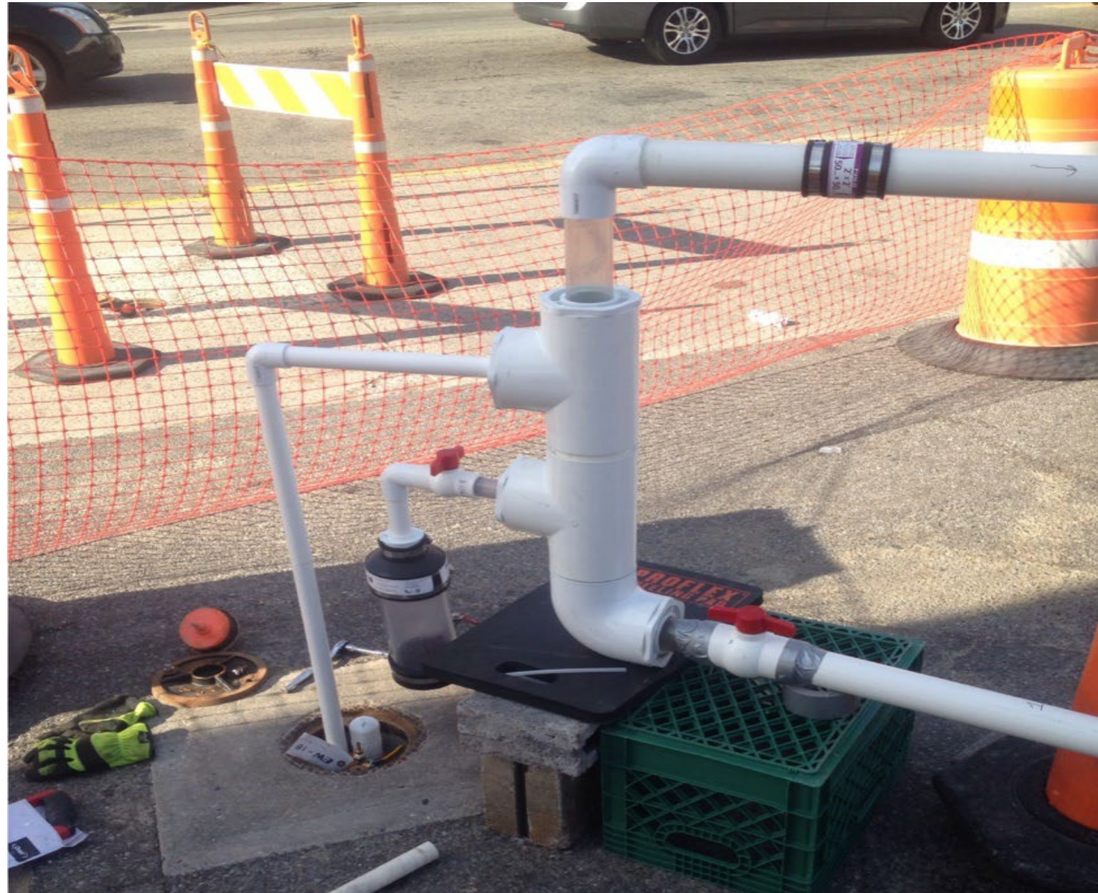
Extraction well head and air/water separation column. Clear 4-inch container was used to measure water flow.
