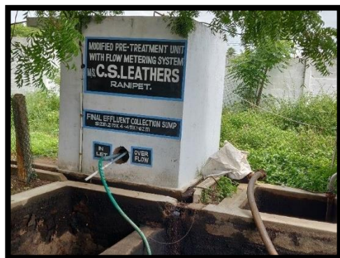
Fig 11: Modified Pre-Treatment Unit in TN
