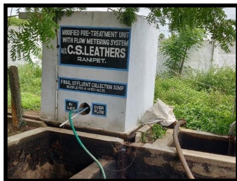
Fig 11: Modified Pre-Treatment Unit in TN
