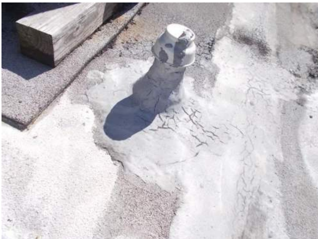
Figure 6.2A-9. One way vent installed within the roof assembly.
