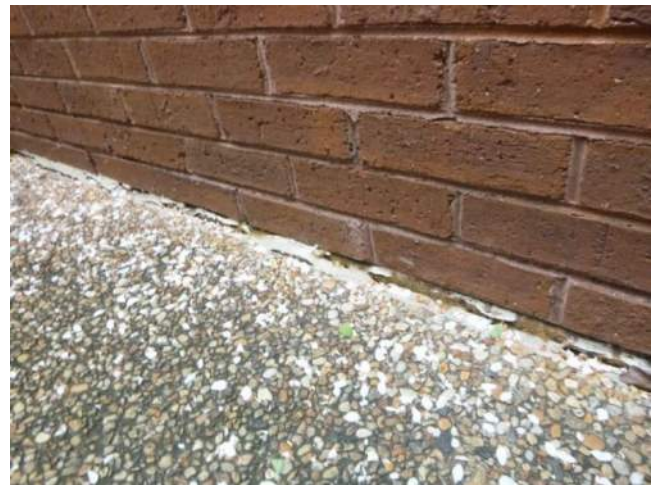
Figure 7.3-2. View of failed sealant at the base of a brick masonry site wall.
