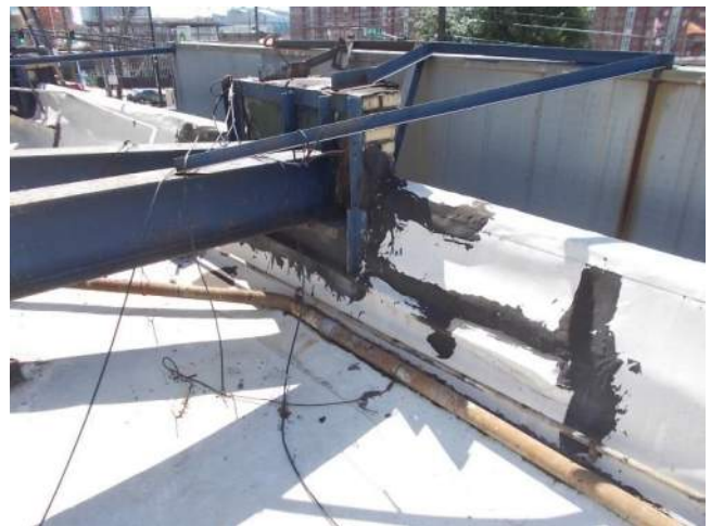
Figure 6.2C-4. Black liquid membrane used to seal the penetration in poor condition.
