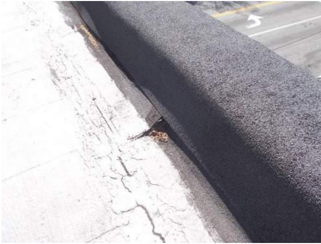
Figure 6.3-17. Open lap seams in the GSMB base flashings.
