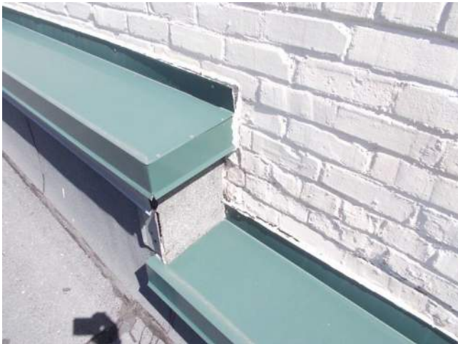
Figure 6.2D-9. Numerous failures in the sealant at the interface of the metal coping and brick wall.
