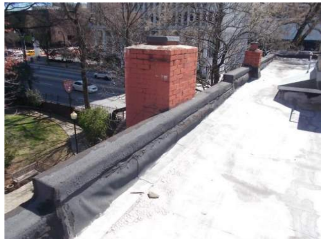
Figure 6.3-14. Multiple wrinkles and blisters in the GSMB base flashings.
