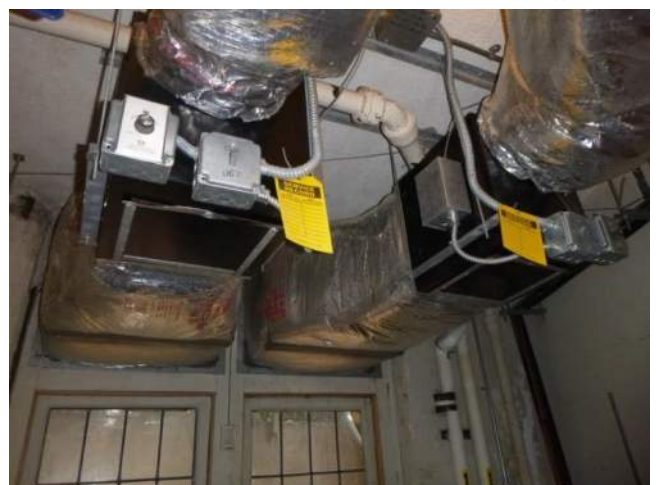
Figure 3.4-6. View of ventilation fans in a storage room adjacent to the music room of Egleston Hall.
