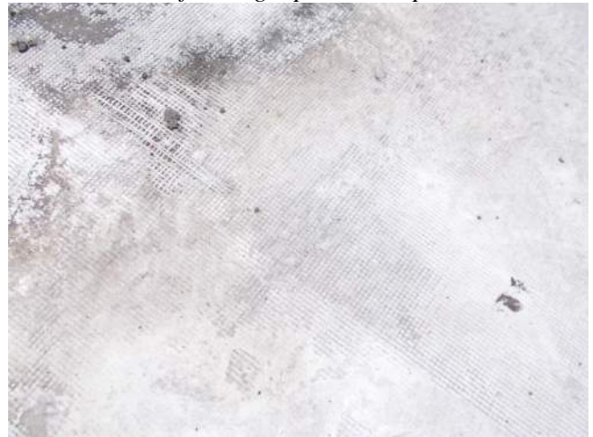
Figure 6.2C-8. Membrane in poor condition as the top surface of the membrane was worn away exposing the fiberglass scrim.
