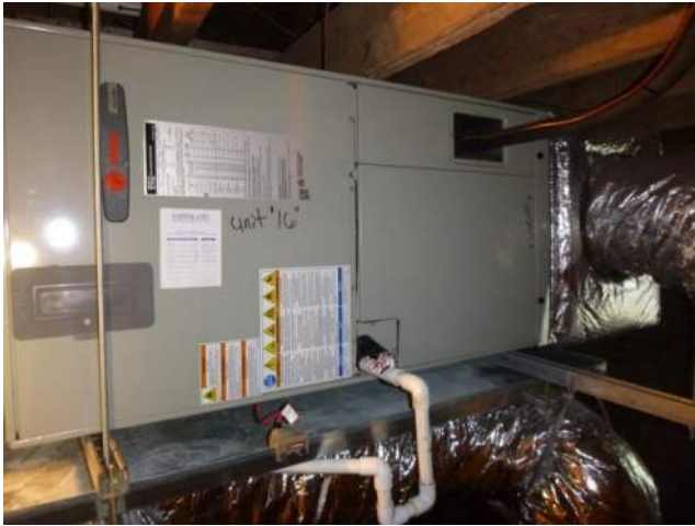
Figure 3.4-7. View of an air handling unit in the attic of Egleston Hall.
