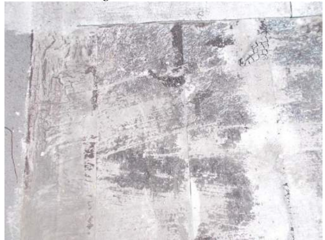
Figure 6.3-8. Weathered, deteriorated, and faded aluminum coating.
