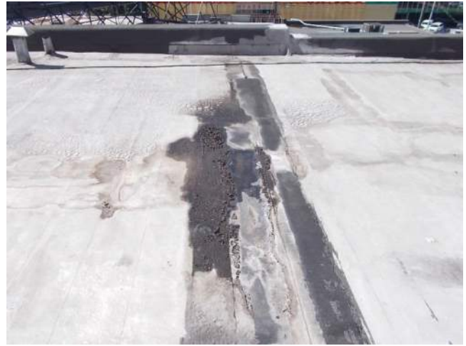
Figure 6.3-18. Cracked patch in the liquid membrane installed along the edges creating an area of ponding water.
