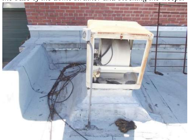
Figure 6.2A-12. Abandoned rooftop equipment with no covers on one of the fans mounted on the equipment curbs.
