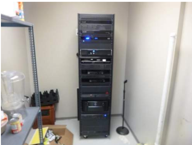
Figure 5.4-37. View of network equipment on the third floor adjacent to the kitchen.
