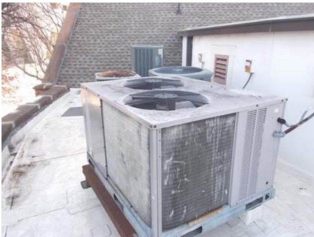
Figure 3.4-9. View of a 7.5 ton RTU at the roof level of Egleston Hall.
