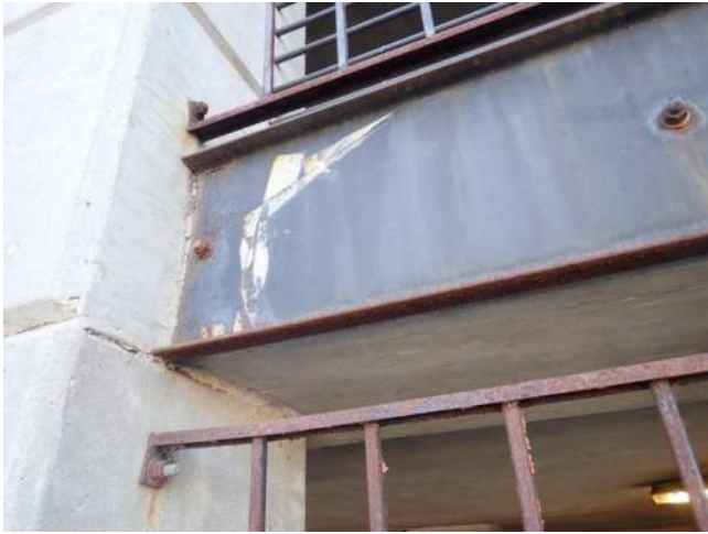
Figure 5.2-13. The existing coating was failed and flaking and in poor condition on the exposed steel elements.
