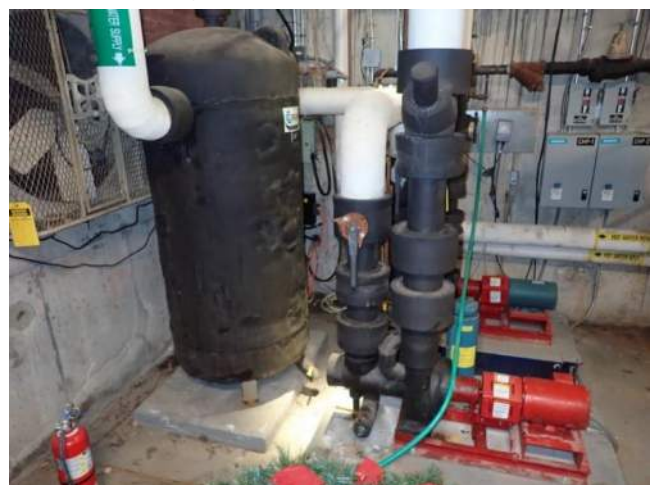
Figure 2.4-6. View of the chilled water buffer system for the main chiller.
