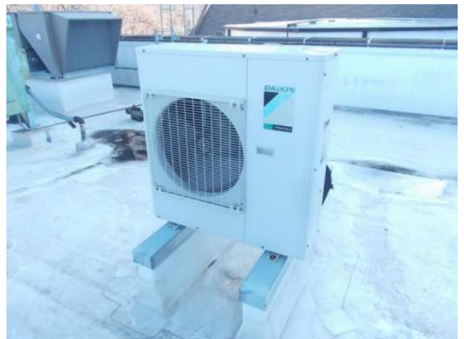
Figure 4.4-6. View of a condensing unit for the Church and Chapel.
