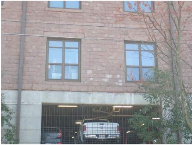
Figure 5.2-7. White haze on the face of the masonry.
