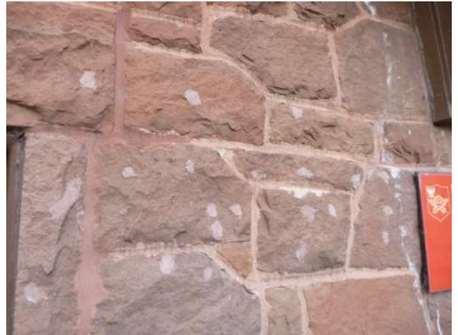
Figure 3.2-8. View of previous bag grouting and remedial spot repair efforts on the Egleston building.
