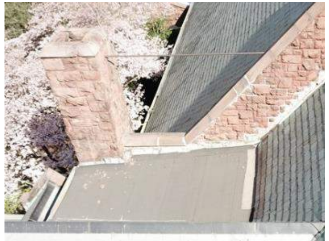
Figure 2.1-22. Coping sealant joints were in poor condition and repair attempts appear to have been implemented.
