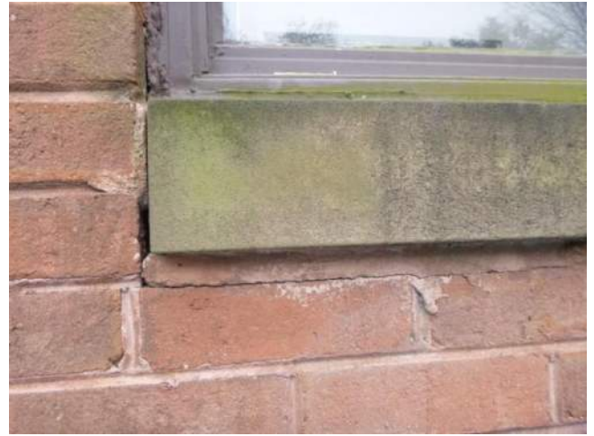
Figure 4.2-12. View of failed and missing mortar at a typical cast stone sill.
