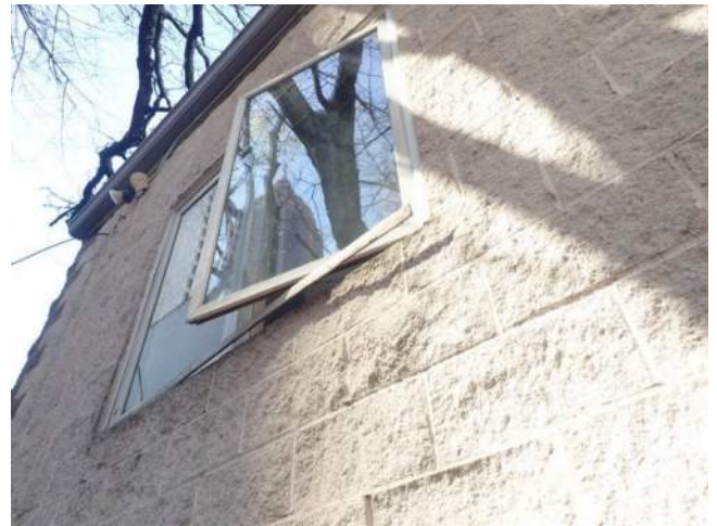
Figure 6.4-2. Isolated damage or displacement in the window trim elements
