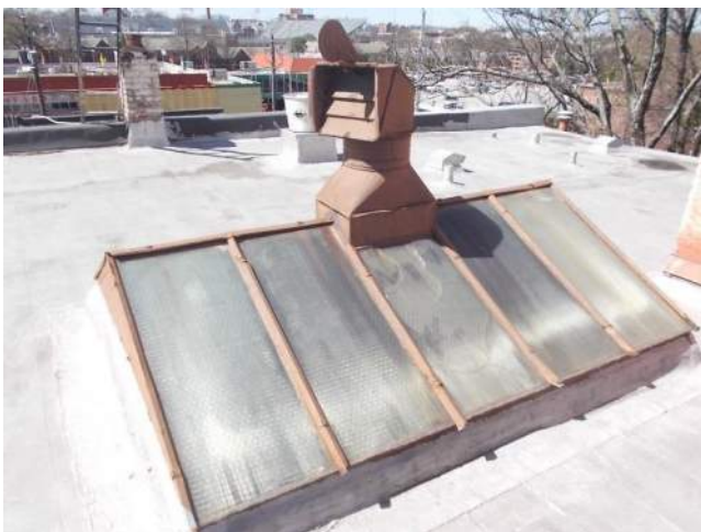
Figure 6.3-19. Weathered, deteriorated and cracked sealants on the skylight with a cracked glass pane.
