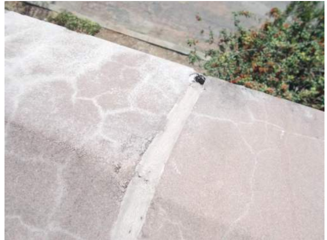
Figure 5.1-10. Cast stone coping with crazing cracks and deteriorated sealant joints.
