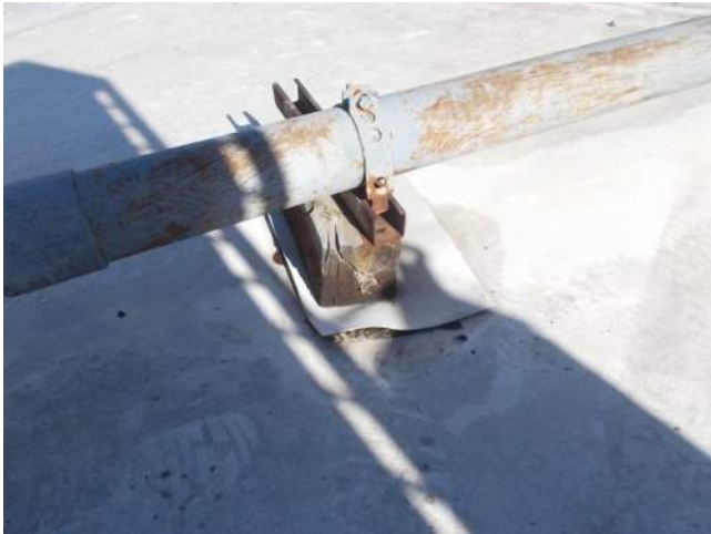
Figure 4.1-15. Wood blocking crushing the underlying roof insulation.
