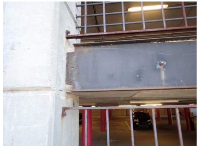
Figure 5.3-12. View of corrosion on metal fencing between openings in the parking structure.
