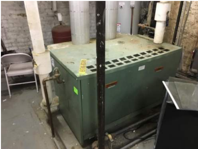
Figure 3.4-1. View of the boiler in the boiler room of Egleston Hall.
