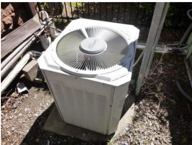
Figure 2.4-3. View of a condenser unit for the Church and Chapel.
