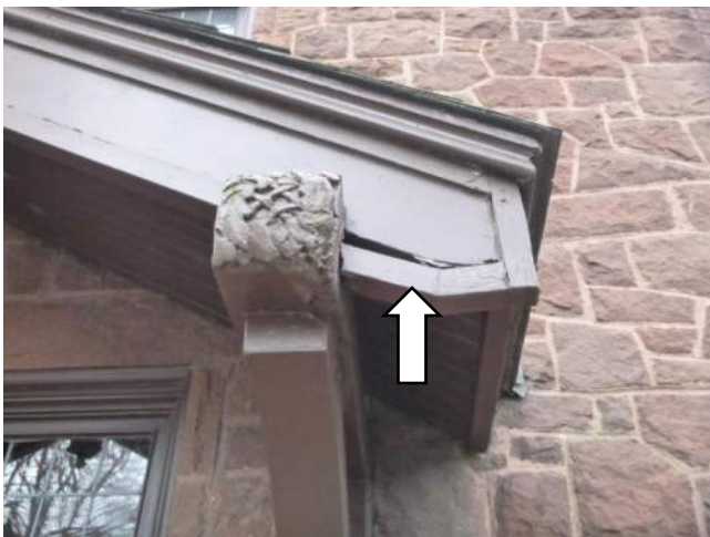
Figure 3.2-21. View of a displaced piece of wood trim at the covered north entrance of the Egleston building.
