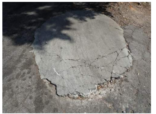
Figure 7.4-611. View of a failed patch repair at the rear entrance drive.
