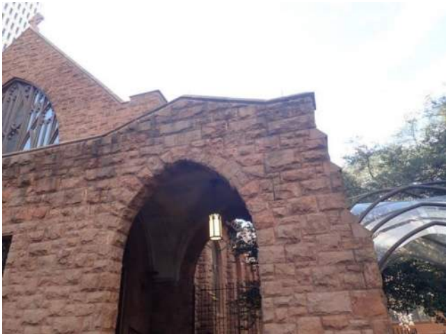
Figure 2.2-9. Face spalls and incipient face spalls located immediately above pedestrian entrance.
