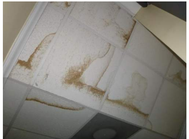
Figure 3.3-34. View of water damaged ceiling panels in a third floor space of the Egleston Building.
