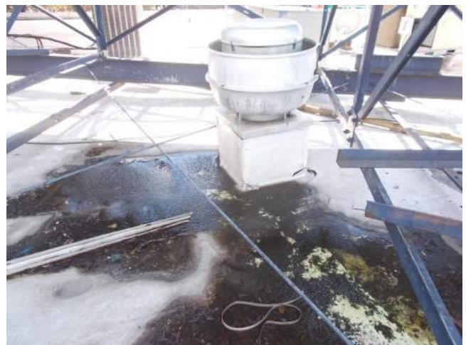
Figure 6.2C-10. Area of ponding water on the roof.
