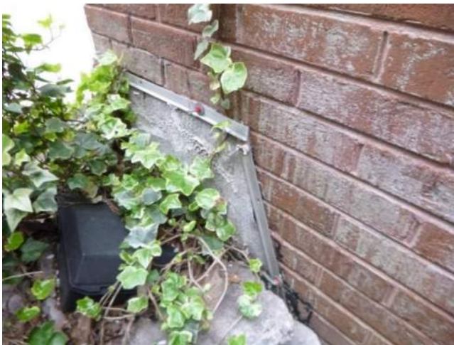
Figure 4.2-9. View of an isolated area of efflorescence on the west elevation.
