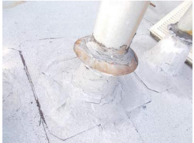
Figure 6.2A-8. View of deteriorated sealant at a pipe penetration.
