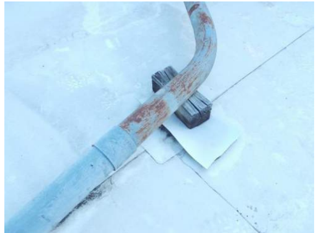
Figure 4.1-12. Mechanical pipes supported with a wood blocking.
