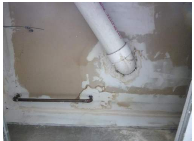
Figure 6.5-6. View of damages to the interior finishes of Tate Hall.
