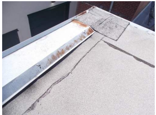
Figure 6.1-6. Small GSMB patch installed at the interface of the edge metal and coping. Note that patch is split.
