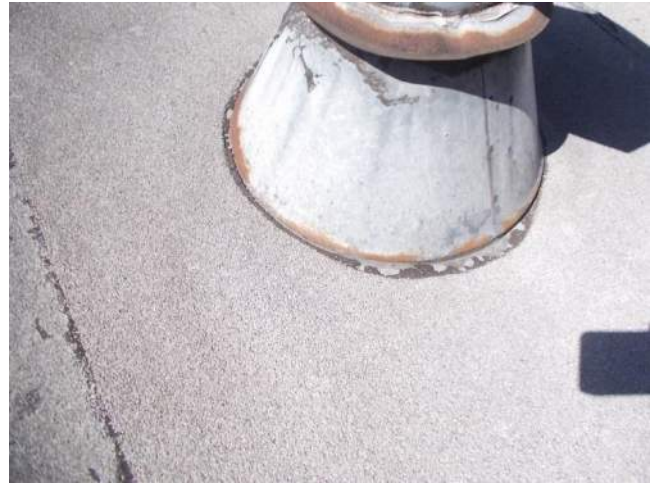
Figure 6.1-8. Deteriorated liquid membrane and sealant at pipe and vent penetrations.
