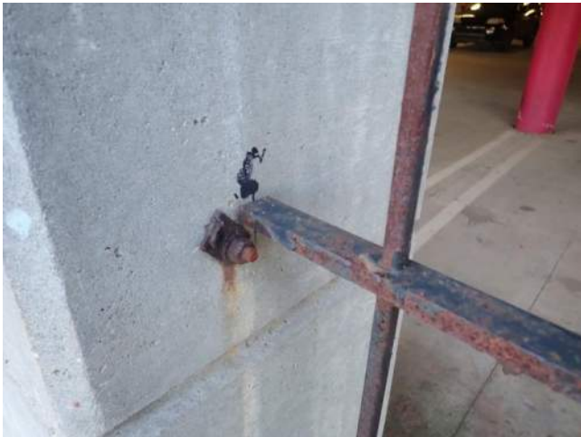
Figure 5.2-9. Failed connections at parking garage fencing.
