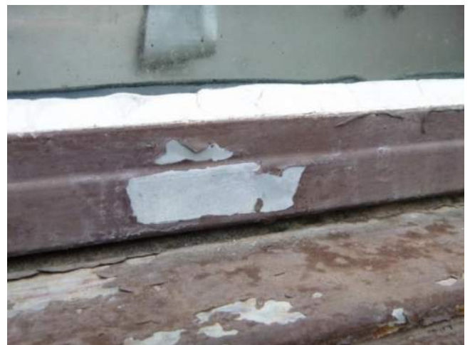
Figure 4.2-16. View of failed painted coating on a window assembly.
