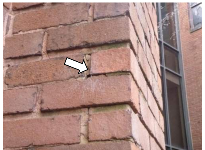
Figure 3.2-12. View of deteriorated mortar joints on the face of a buttress on Egleston Hall.
