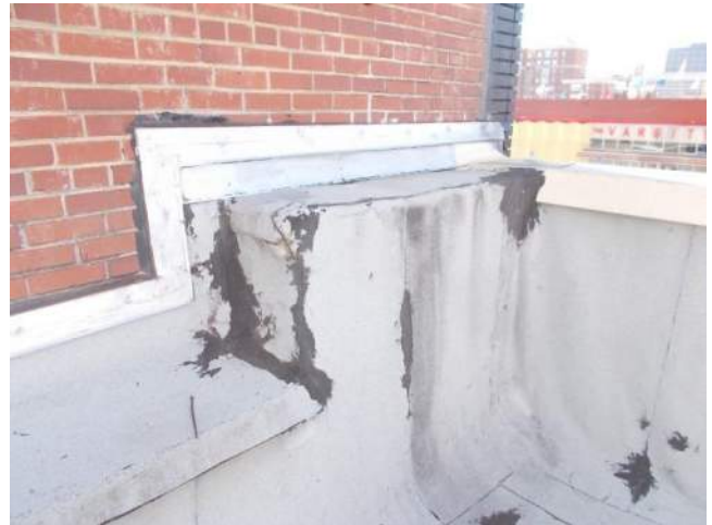
Figure 6.2A-4. Liquid membrane patches and apparent repair attempts.
