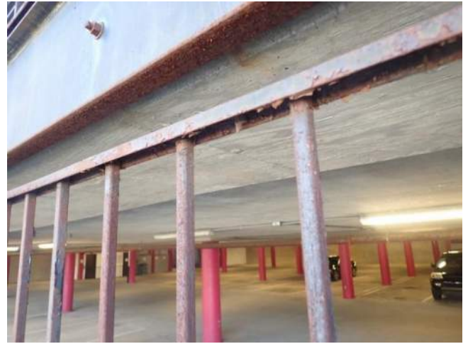
Figure 5.2-14. Widespread surface corrosion on the steel fencing at the openings in the parking structure.
