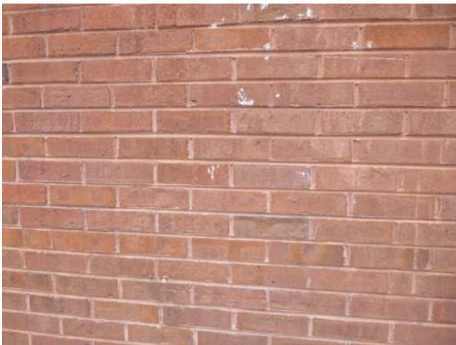
Figure 4.2-1. View of the condition of a typical area of brick masonry facade of the Parish House.
