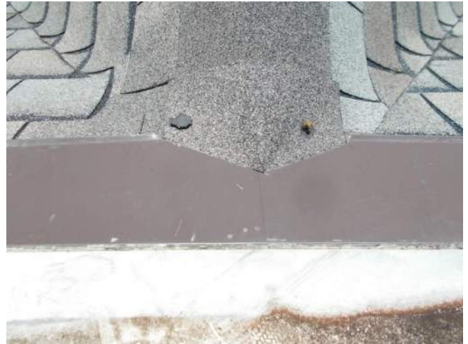
Figure 5.1-22. Exposed nail fasteners in the asphalt shingled roof areas.
