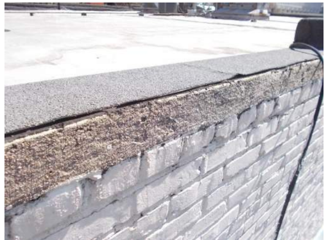
Figure 6.3-10. Wrinkles, fishmouths, and poorly sealed edges of the membrane.
