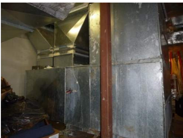
Figure 2.4-5. View of the air handling system for the Chapel building.
