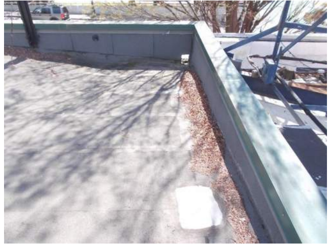
Figure 6.2D-14. Organic debris collecting at the southeast and southwest corners of the roof.
