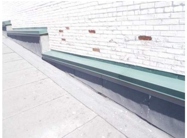
Figure 6.2D-8. Delaminated outer face of numerous brick masonry units with bubbled and flaking coating.
