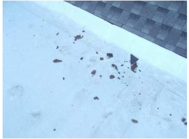
Figure 3.1-10. View of stone debris on the low slope roof portion of Egleston Hall.
