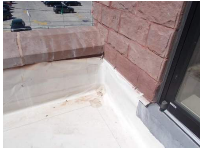
Figure 5.1-12. Expansion joint in the outer wall at the northwest corner of the roof does not continue up and over the wall to the roof.
