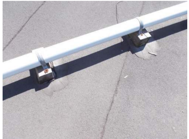
Figure 6.2B-10. Wood blocking pipe supports resting directly on the roof membrane surface with liquid membrane patches under the supports.
