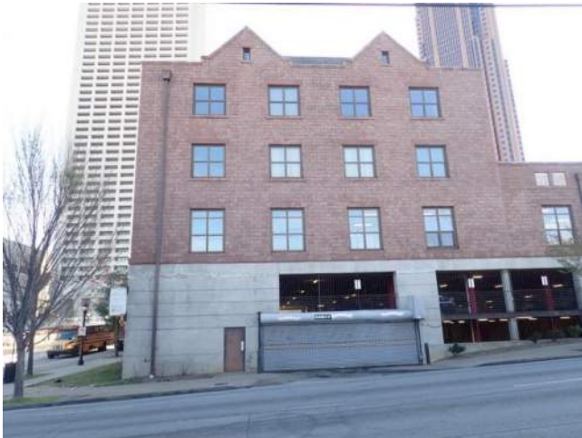
Figure 5.2-3. Overall view of the condition of the manufactured stone masonry facade.
