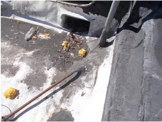
Figure 6.2C-5. Black liquid membrane used to seal the membrane lap seams in poor condition.
