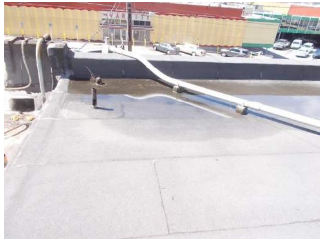
Figure 6.2B-8. Large area of ponding water at the southwest corner of the roof around the area drain.
