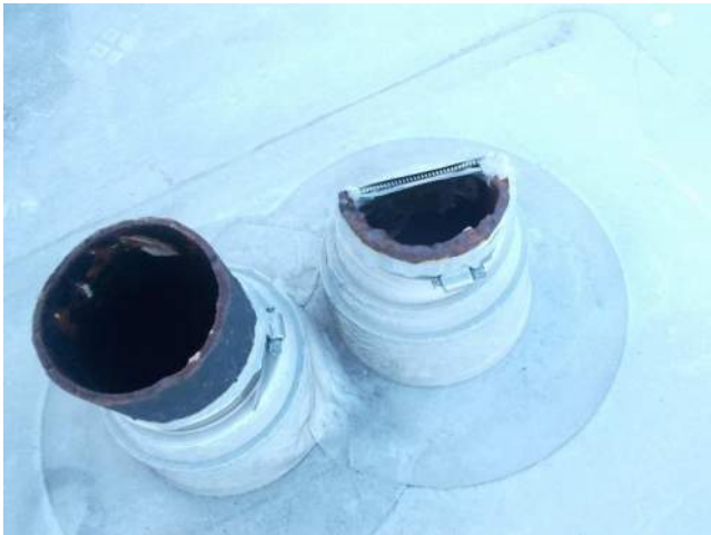
Figure 4.1-11. Broken cast iron pipe penetration.
