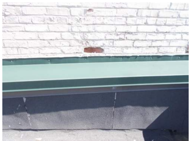
Figure 6.2D-12. Base membrane flashing lap seams contained additional sealant, most likely as an attempt for repair.
