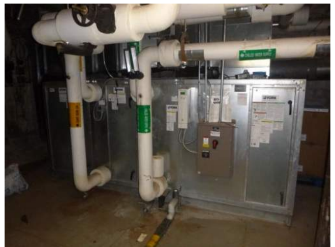
Figure 2.4-4. View of the primary air handler for the Church building.
