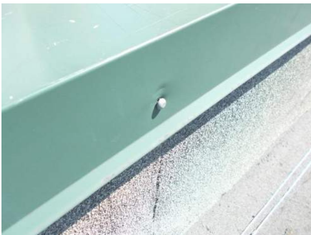
Figure 6.2B-11. Open and unsealed exposed fasteners on the metal coping along the east end of the roof.
