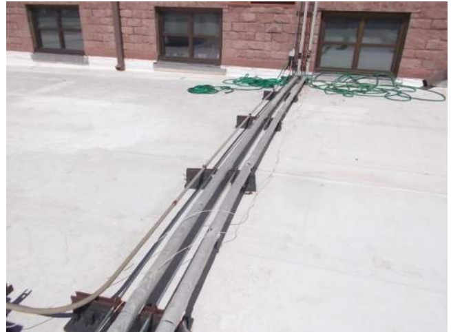
Figure 5.1-4. Mechanical pipes supported with prefabricated supports with integral protection pads.
