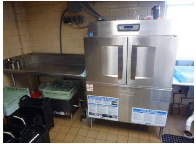
Figure 4.3-10. View of the commercial dishwasher in the Parish House kitchen.
