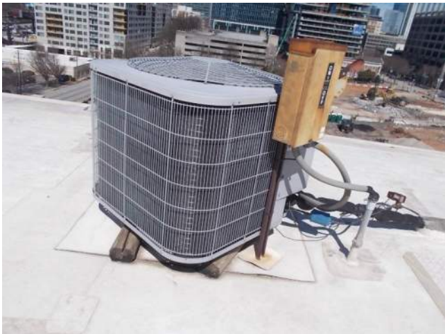
Figure 5.1-23. Wood blocking be crushing the underlying roof insulation as it was depressed into the roof membrane.
