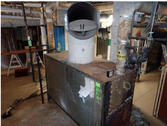
Figure 2.4-9. View of the AJAX boiler system for the Church and Chapel.
