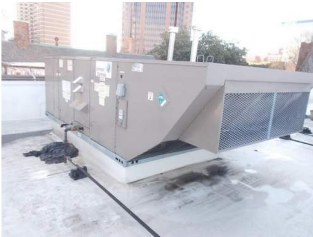
Figure 4.4-3. View of a RTU at the Parish House roof level.
