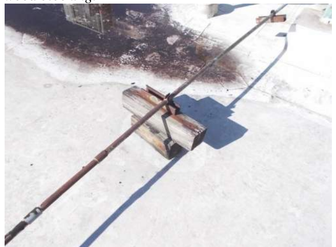
Figure 4.1-14. Wood blocking which did not have membrane protection sheets
