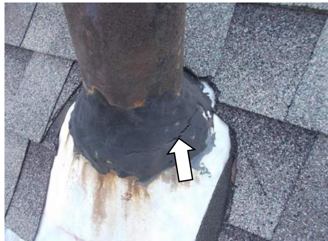
Figure 3.1-18. Weathered and cracked liquid membrane at one of the pipe penetrations.
