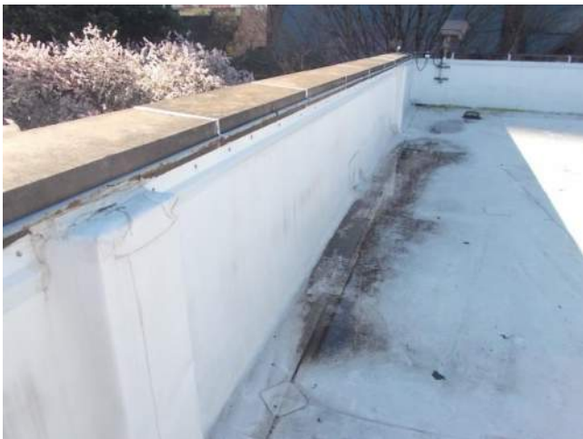
Figure 4.1-5. Ponding water along the parapet wall.
