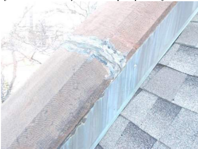
Figure 3.1-13. View of deteriorated sealant repairs at coping.
