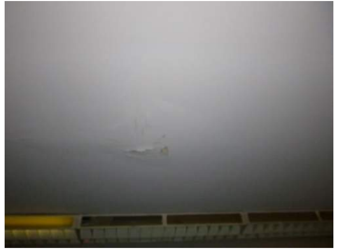
Figure 6.5-8. View of water damage to a ceiling finish in Tate Hall.
