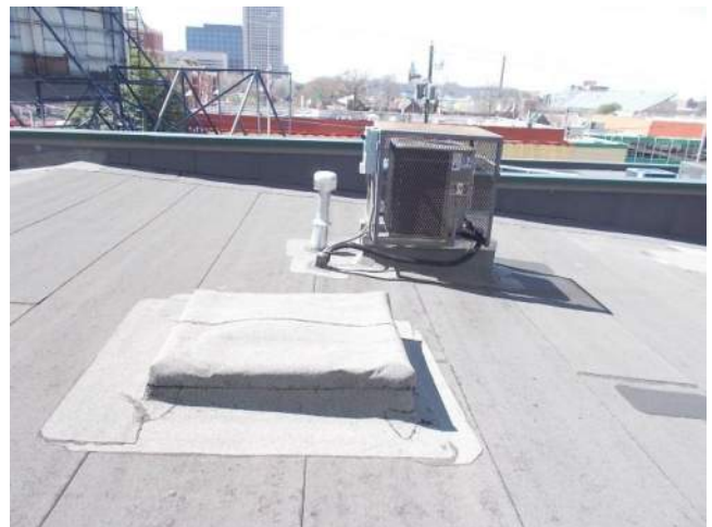
Figure 6.2D-6. Patches at what appeared to be abandoned equipment curbs.
