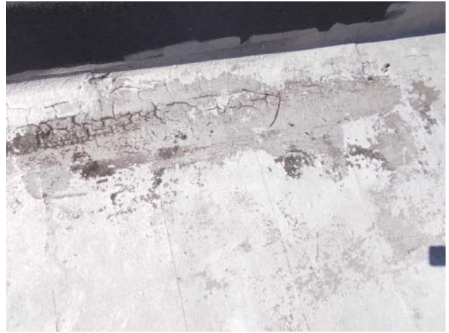
Figure 6.3-6. Weathered, deteriorated, and faded aluminum coating.
