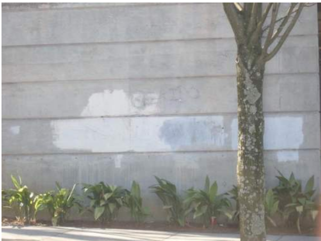
Figure 5.2-15. Evidence of graffiti at the northeast corner of the parking structure
