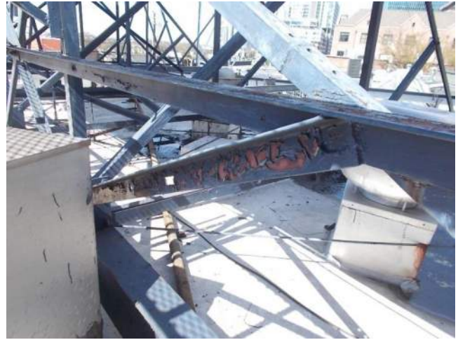
Figure 6.2C-18. Paint on the steel framing for the billboard is in poor condition and is flaking and peeling off of the substrate.
