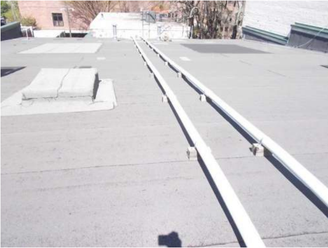
Figure 6.2D-13. Wood blocking pipe supports resting directly on the roof membrane surface.
