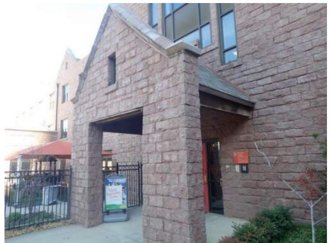
Figure 5.2-18. Wood trim and soffit at the entrance canopy at the southeast entrance had been removed, exposing the wood structural framing elements.
