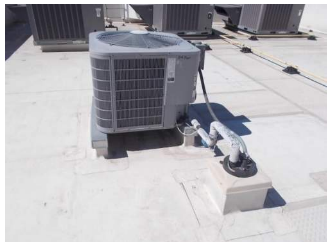
Figure 5.5-6. View of an RTU on the upper roof of the Pritchett Center.
