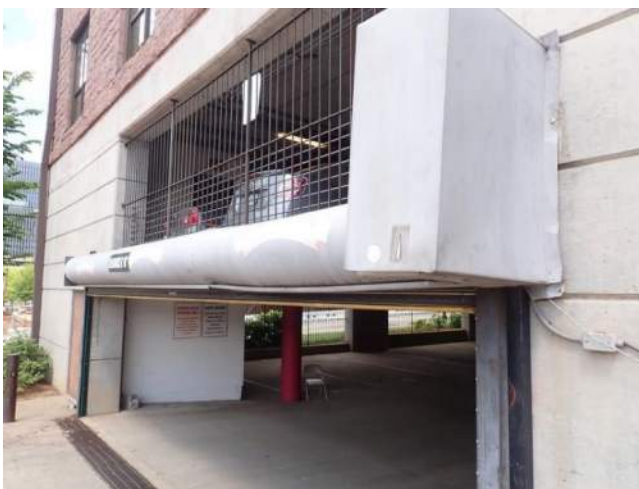
Figure 5.3-5. View of an overhead door and control motor at the Spring Street entrance.
