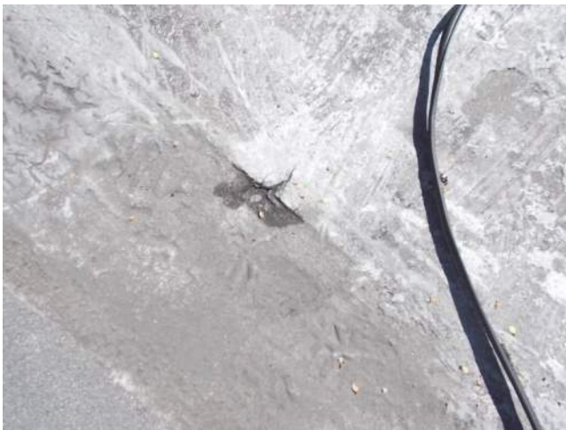
Figure 6.3-13. Split in the membrane with moisture extending from the split.
