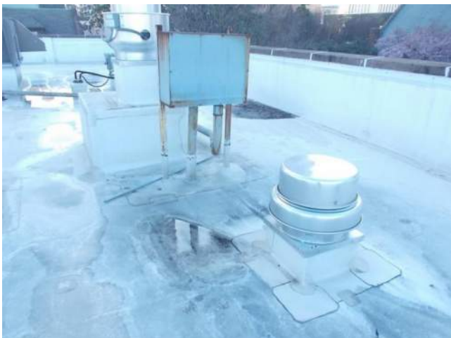
Figure 4.4-5. View of an exhaust fan on the Parish House roof.
