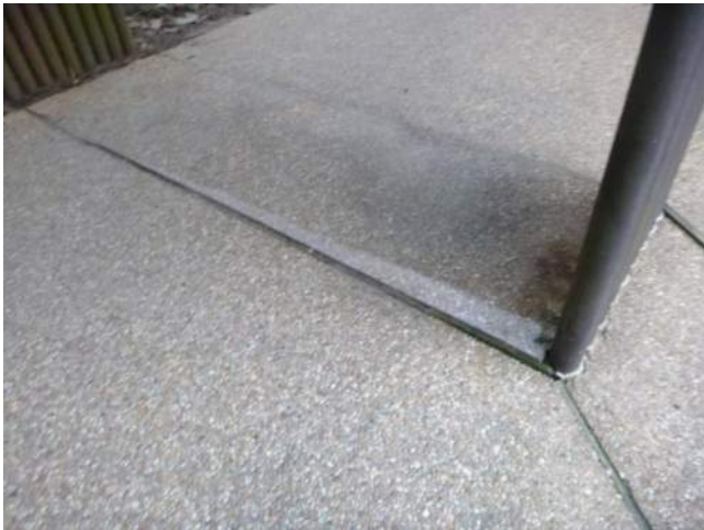
Figure 7.2-33. View of vertical displacement of a section of cast walkway near Egleston Hall.
