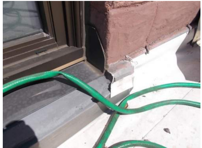
Figure 5.1-6. Through wall flashing interfaces the window opening and is not well sealed or integrated.
