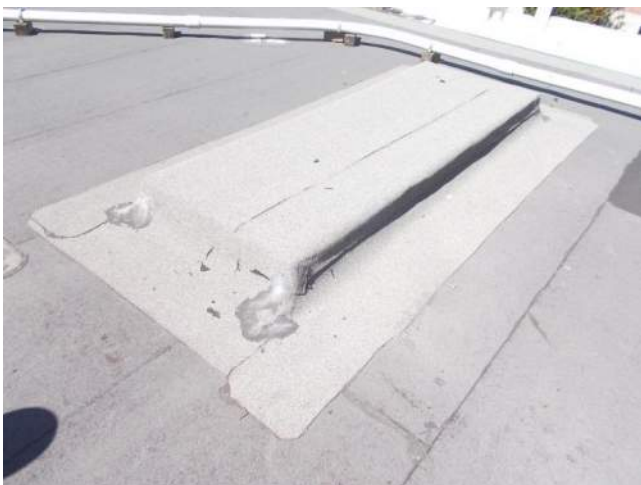
Figure 6.2B-5. Patch on the roof near an abandoned equipment curb.
