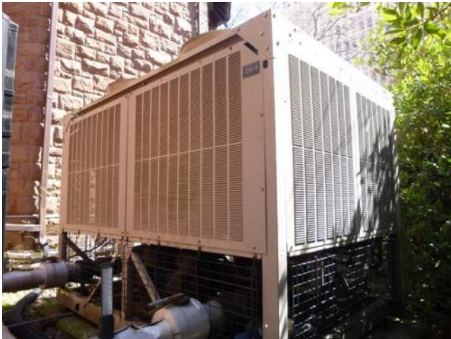
Figure 2.4-1. View of the main chiller for the Church and Chapel.
