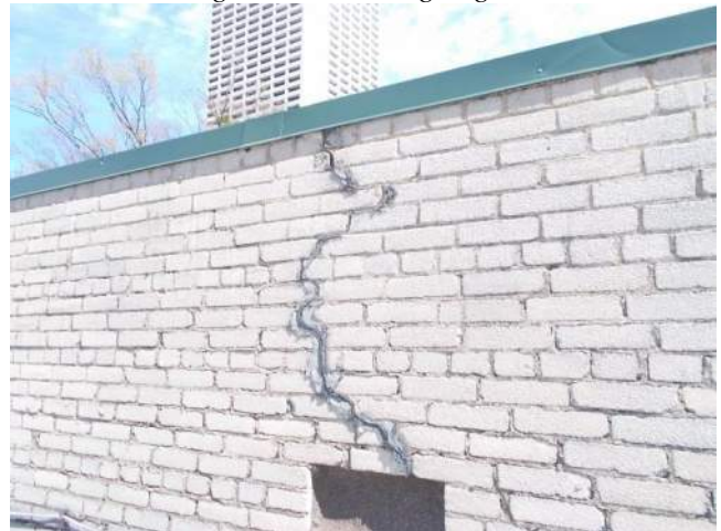
Figure 6.2C-14. Large cracks in the adjacent brick masonry wall.
