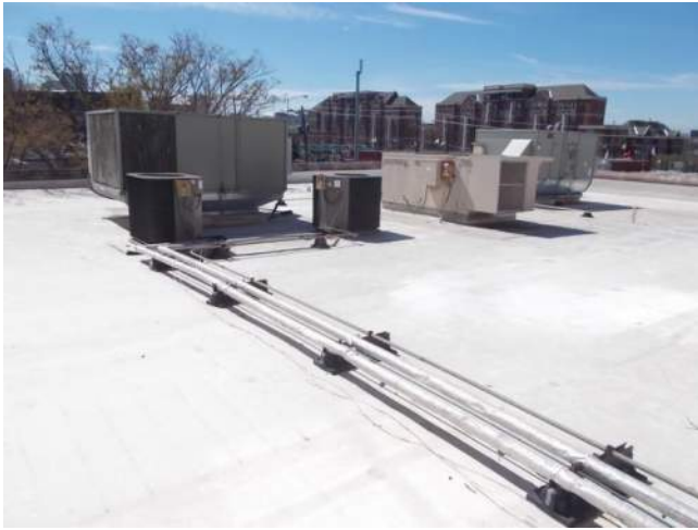
Figure 5.5-7. View of mechanical equipment on the lower roof of the Pritchett Center.
