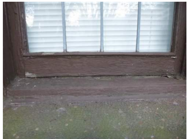
Figure 3.2-18. View of typical condition of wood window surrounds on the Egleston building.
