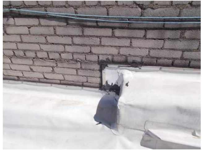
Figure 6.2C-12. Roof membrane contained liquid membrane along the terminating edge.
