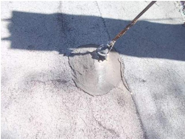
Figure 6.2D-7. Penetration contained weathered, deteriorated and cracked liquid membrane seals.
