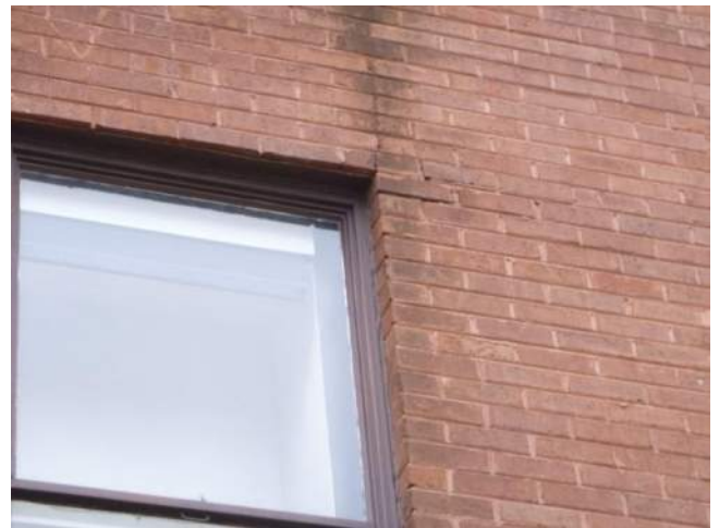
Figure 4.2-4. View of deteriorated mortar at a window corner.
