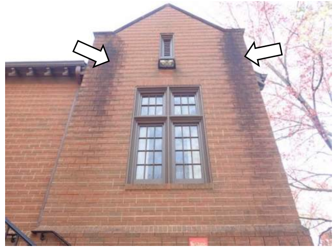
Figure 2.2-20. Accumulation of atmospheric staining and soiling on the brick masonry veneer.
