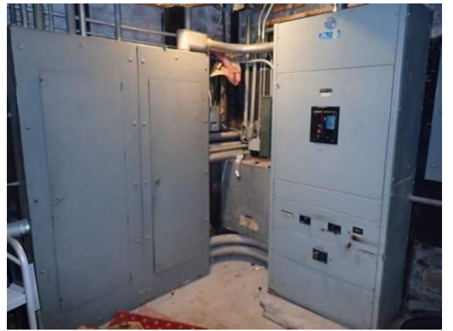
Figure 2.4-10. View of the main service panels and switchboards in the basement level.
