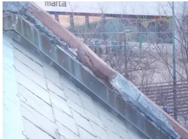
Figure 3.1-12. View of previous mortar and liquid membrane repairs on the terra cotta coping.
