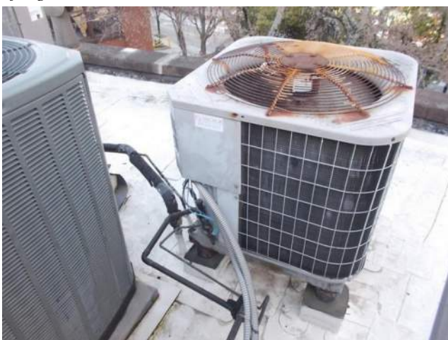
Figure 3.4-11. View of additional split heat pumps at the roof level of Egleston Hall.
