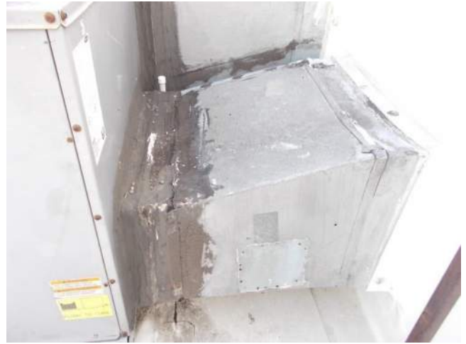
Figure 3.1-16. Failed sealant between the HVAC units and the exposed ductwork.
