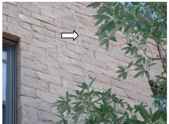
Figure 5.2-6. Weathered sealant within the expansion joint.
