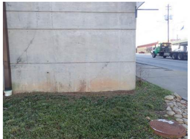
Figure 5.2-12. Isolated cracking at the northwest corner of the parking garage.
