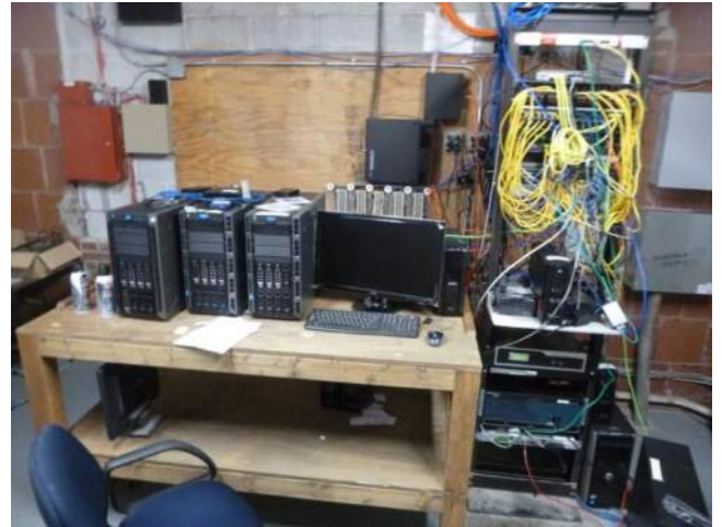
Figure 4.4-8. View of the engineer's office and building system controls.
