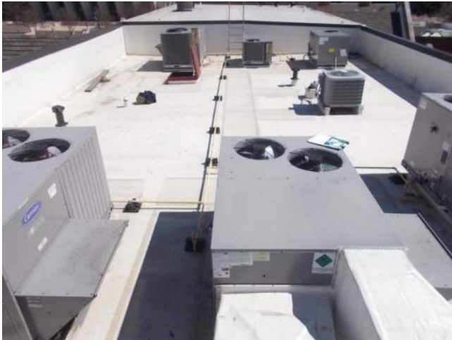
Figure 5.5-1. View of mechanical equipment on the upper roof of the Pritchett Center.
