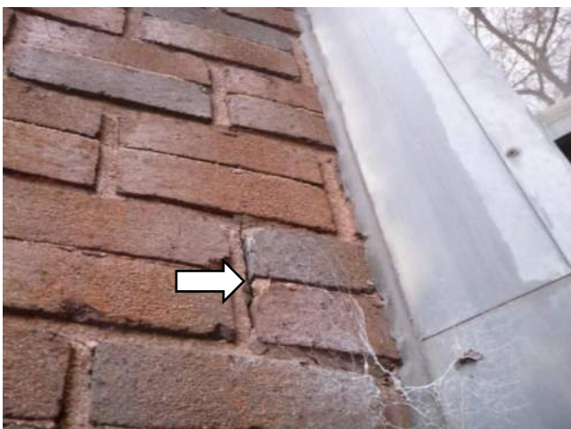
Figure 3.2-11. View of a failed mortar joint in an area of brick masonry on the Egleston building.
