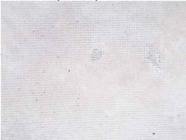
Figure 6.2C-7. Membrane in poor condition as the top surface of the membrane was worn away exposing the fiberglass scrim.
