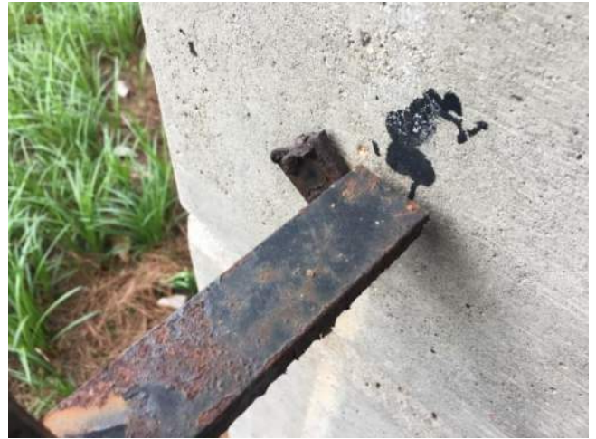
Figure 5.3-8. View of a failed connection in the metal fencing.
