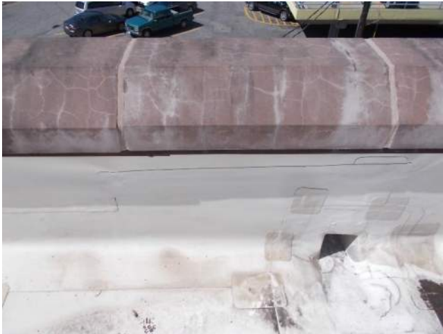
Figure 5.1-9. Cast stone coping with crazing cracks and deteriorated sealant joints.
