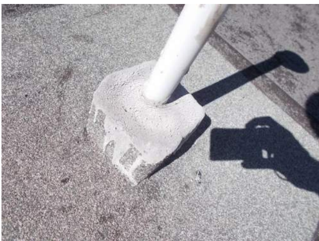
Figure 6.2D-11. Pitch pocket fillers and liquid membrane seals at penetrations are weathered, deteriorated and cracked.
