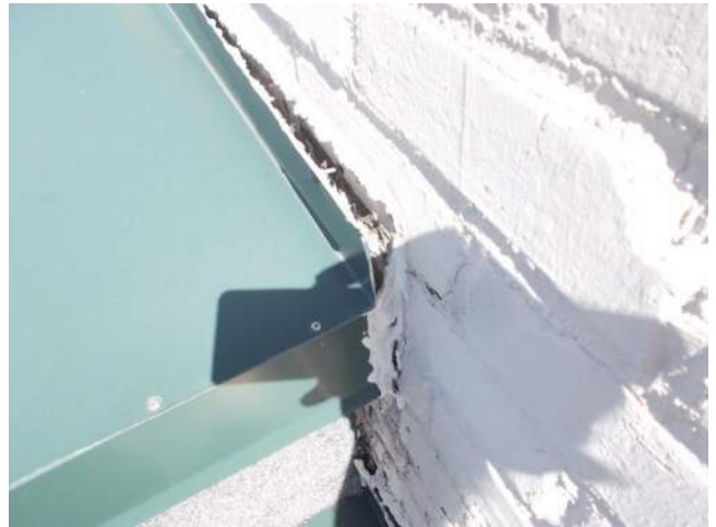
Figure 6.2D-10. Numerous failures in the sealant at the interface of the metal coping and brick wall.
