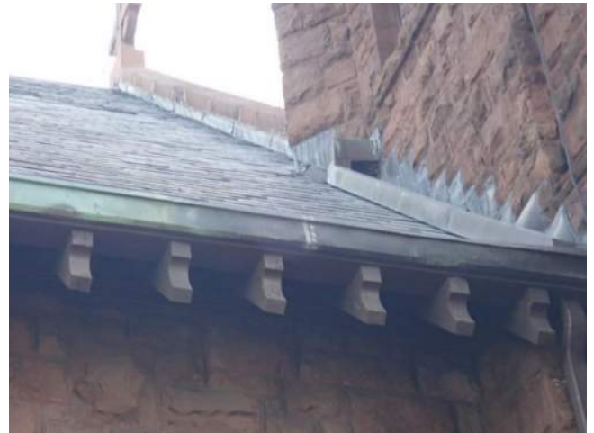
Figure 2.2-28. Weathered and flaking coating on the wood elements.
