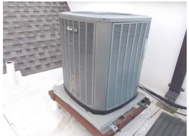
Figure 3.4-10. View of a heat pump at the roof level of Egleston Hall.
