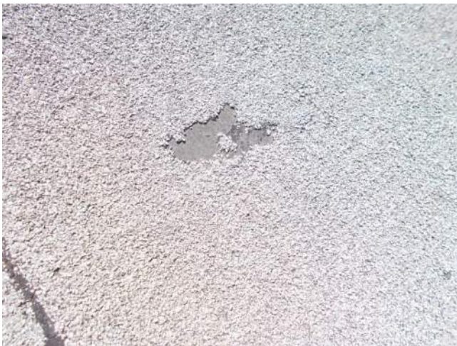
Figure 6.1-5. Isolated area with significant granule loss.
