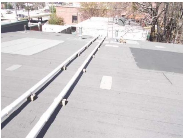
Figure 6.2D-5. Multiple GSMB membrane and liquid membrane patches throughout the roof area.
