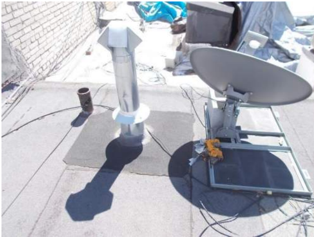
Figure 6.2B-7. Rooftop equipment resting directly on the roof membrane with no protection pads.
