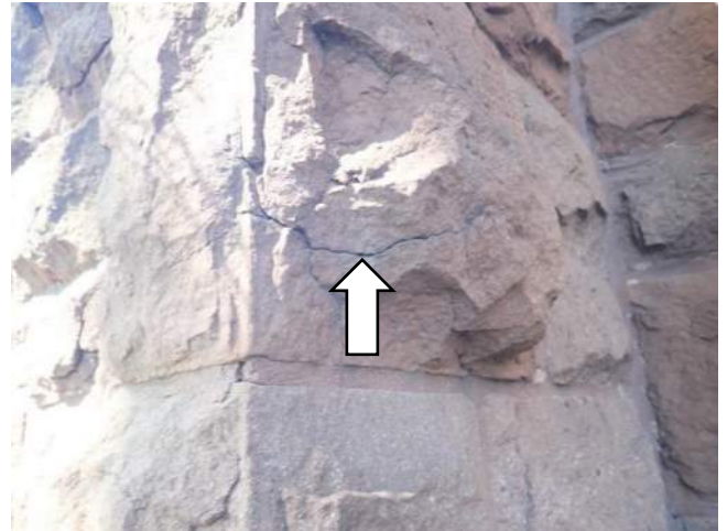
Figure 2.2-8. View of delamination of the face of a sandstone unit.
