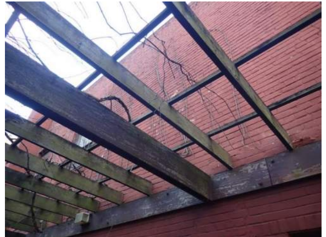
Figure 6.4-12. Vegetation growing on the surface of the facade at the east facade.
