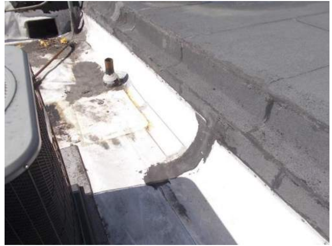
Figure 6.2C-6. Black liquid membrane used to seal the membrane base flashing lap seams in poor condition.
