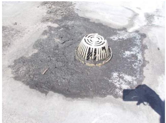
Figure 6.2A-10. Organic debris accumulating around the base of the dome strainer and blocking the weeps.
