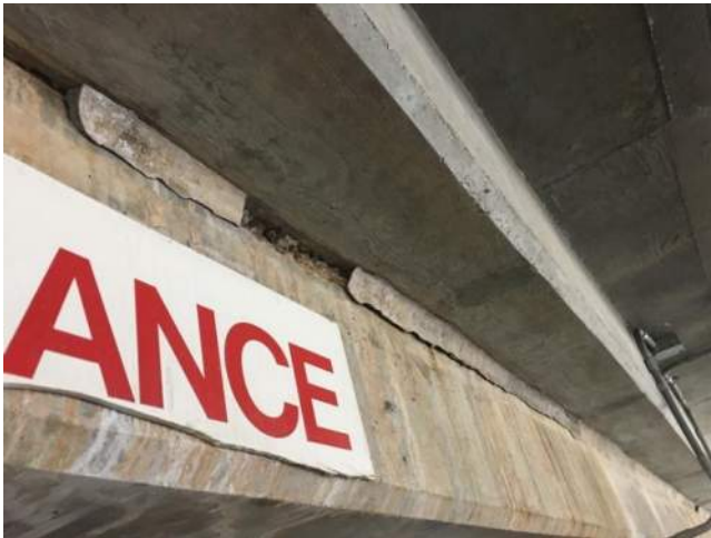
Figure 5.3-3. View of loose overhead concrete in parking garage from original formwork.
