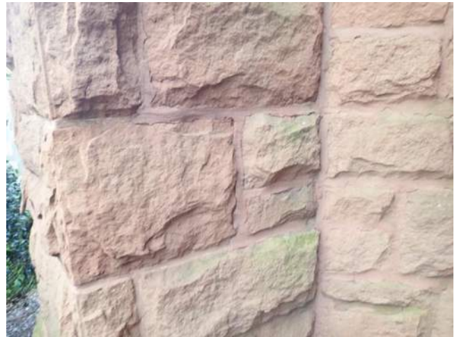
Figure 2.2-4. Three different mortar colors indicate at least two separate repair efforts during the life of the building.
