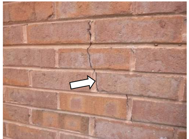
Figure 4.2-2. View of a stepped crack in the brick masonry facade of the Parish House.
