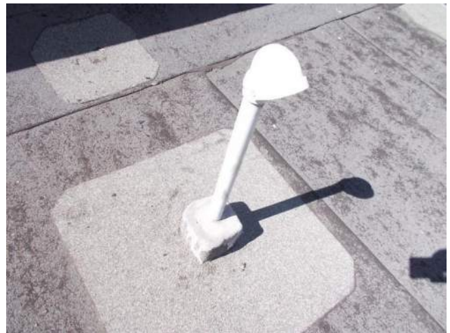
Figure 6.2D-4. Moderate granule loss on the membrane, mostly near the north end of the roof.
