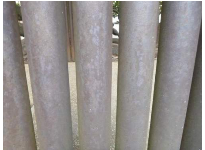
Figure 7.2-4. View of atmospheric soiling on the coating and light surface corrosion of the steel tubing.
