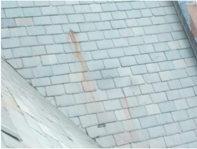
Figure 3.1-9. View of area of typical staining on the slate tile roof portion of Egleston Hall.
