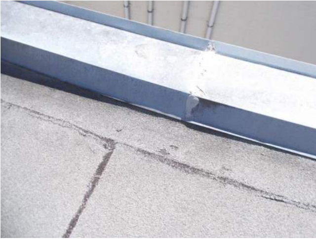
Figure 6.1-7. Weathered sealant at the lap or splice joints in the metal coping.
