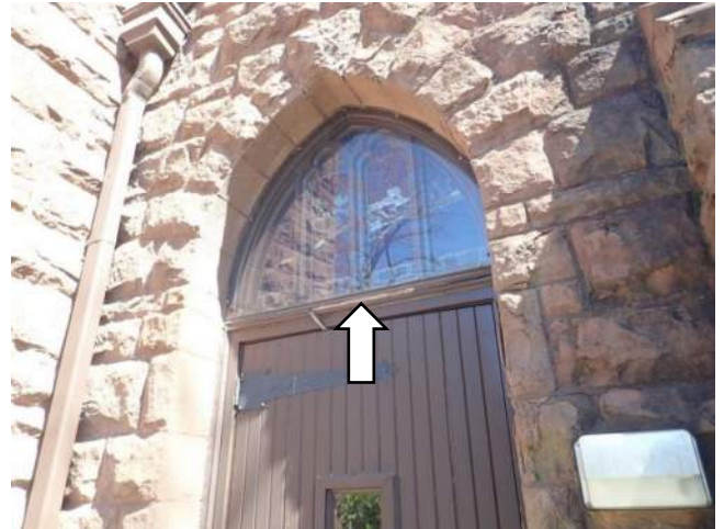
Figure 2.2-26. Wood door at the west facade in good to fair condition; with flaking paint.
