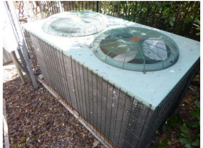
Figure 2.4-2. View of a condensing unit for the Church and Chapel.
