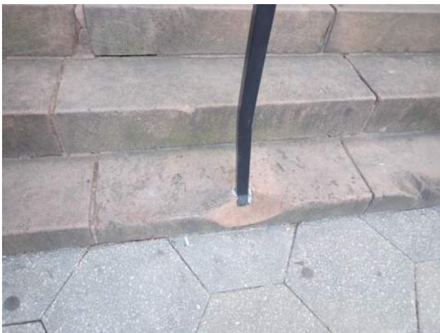
Figure 7.1-5. View of a damaged handrail at the main Church building.
