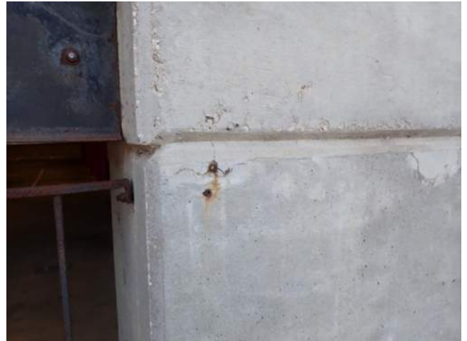
Figure 5.2-14. Surface cracking and shallow surface spalls at the north elevation.
