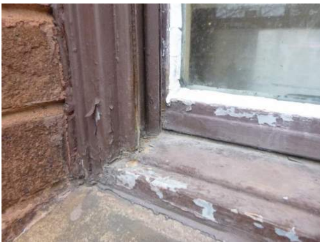
Figure 4.2-15. View of failed painted coating on a window assembly.
