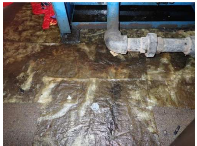
Figure 5.6-2. View of the leak in the elevator hydraulic system.
