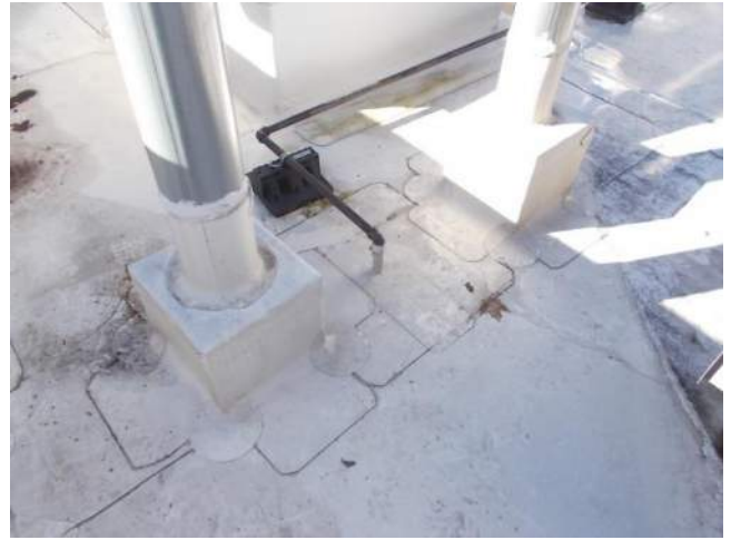
Figure 4.1-10. Membrane penetration flashings at equipment curbs and pipe penetrations.
