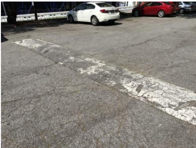
Figure 7.4-3. View of the condition of the asphalt paving of the parking area.
