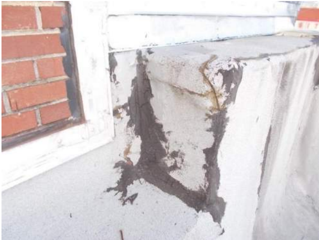
Figure 6.2A-7. View of cracked liquid membrane patches.
