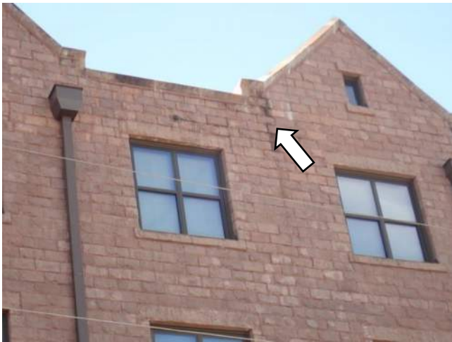
Figure 5.2-9. Atmospheric soiling beneath the sloped portion of the coping units at the gabled ends.
