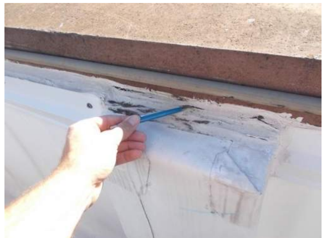
Figure 4.1-8. View of failed sealant at the top of the piers at the interface of the metal counter flashing.
