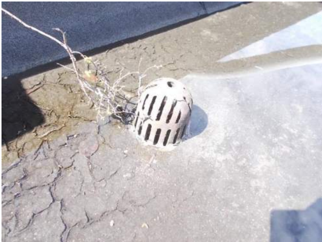
Figure 6.2B-9. Organic debris accumulated around the base of the drain strainer preventing proper drainage of the water on the roof surface.
