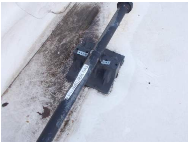
Figure 4.1-13. Mechanical pipes supported with a prefabricated supports.
