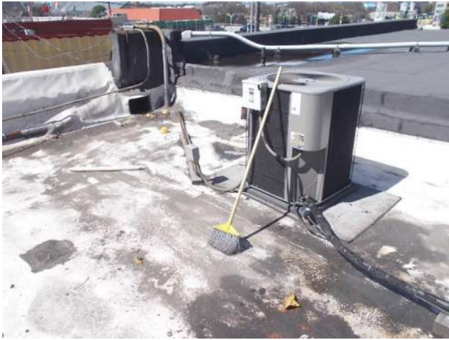
Figure 6.2C-11. Signs of ponding water along the northwest corner of the roof.
