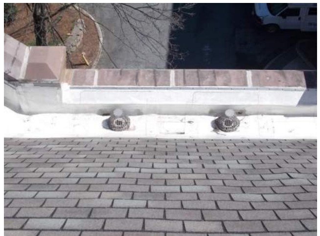
Figure 5.1-20. TPO roof membrane at internal gutter terminated with mechanically fastened termination bars and sealant.
