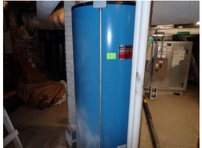
Figure 2.4-8. View of the 200 gallon hot water storage tank.
