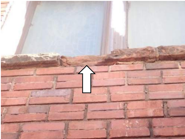
Figure 2.2-15. Spall in the granite unit at sill.
