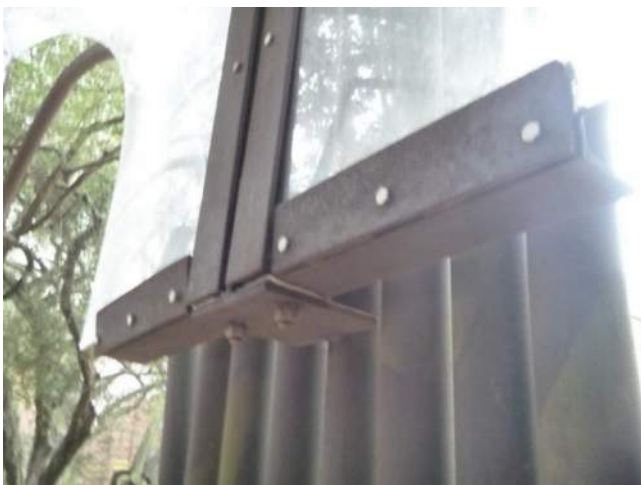
Figure 7.2-5. View of light surface corrosion and soiling on the canopy structure.
