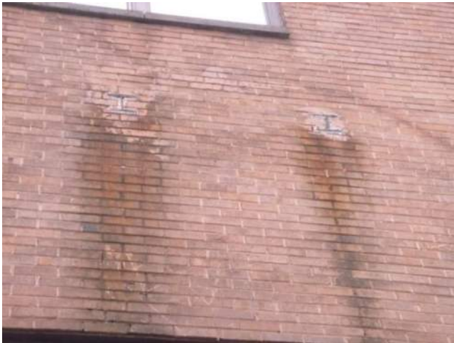
Figure 4.2-7. View of staining from embedded steel in the masonry facade on the west elevation.
