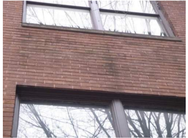
Figure 4.2-6. View of an area of soiling on the brick masonry below a window on the second floor.
