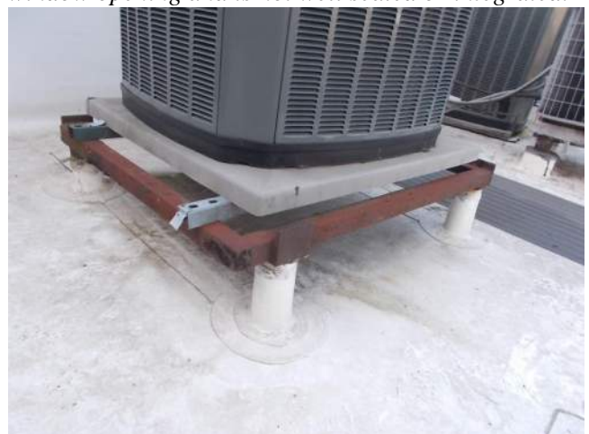
Figure 5.1-8. Equipment curbs flashed with a combination of TPO membrane flashing and prefabricated TPO pitch pockets.
