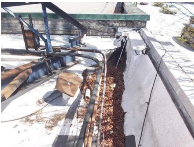
Figure 6.2C-15. Organic and material debris accumulating near the corners of the roof
