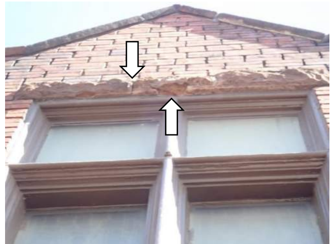
Figure 2.2-16. Cracks and spalls in the granite units at window head.
