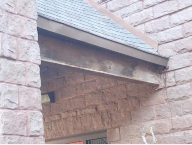
Figure 5.2-19. Water staining on the exposed structural members.
