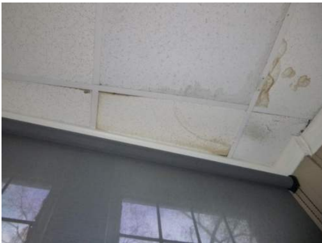
Figure 3.3-33. View of water damaged ceiling panels in a third floor office of the Egleston Building.
