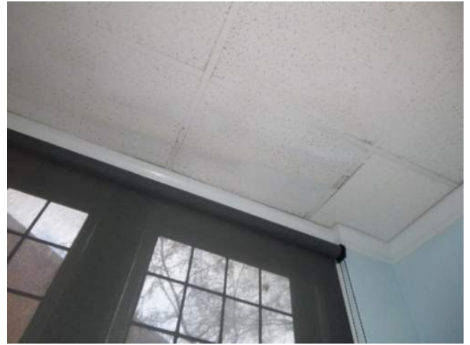
Figure 3.3-32. View of water damaged ceiling panels in a third floor office of the Egleston Building.
