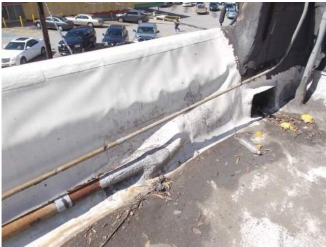
Figure 6.2C-19. Poorly sealed pipe conduit on the wall penetrating the roof membrane
