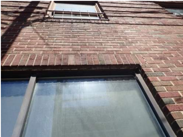
Figure 6.4-11. Light surface corrosion on the steel lintels at openings throughout the building.
