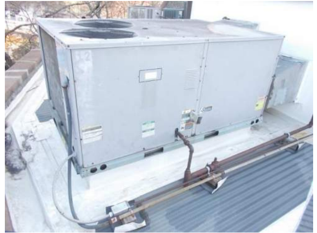
Figure 3.4-8. View of the 8.5 ton RTU at the roof level of Egleston Hall.
