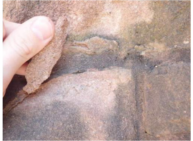
Figure 2.2-2. Deficiencies within the mortar joints between the sandstone units.
