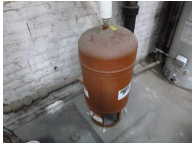
Figure 3.4-2. View of the expansion tank in the boiler room of Egleston Hall.
