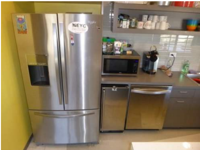
Figure 5.4-35. View of kitchen equipment in the third floor kitchen.
