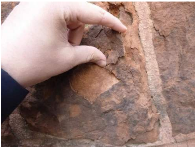
Figure 3.2-9. View of flaking of the exterior face of a sandstone unit on the ground level of the Egleston building.
