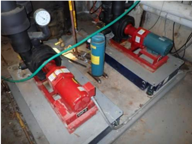
Figure 2.4-7. View of pumps CHP-1 and CHP-2.
