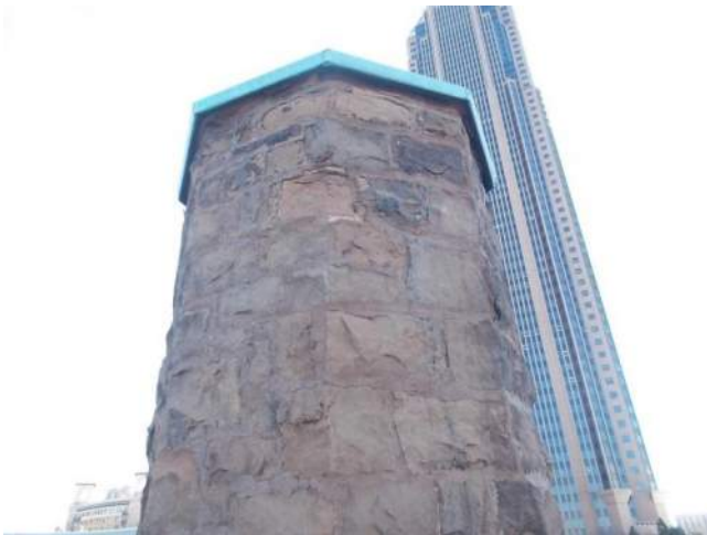
Figure 3.1-11. View of typical delaminated portions of the stone chimneys in the steep sloped roof.
