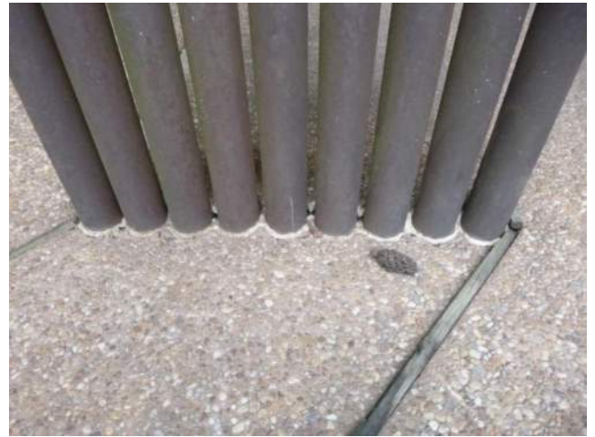
Figure 7.2-2. View of deteriorated sealant at the support post bases on the canopy structure.
