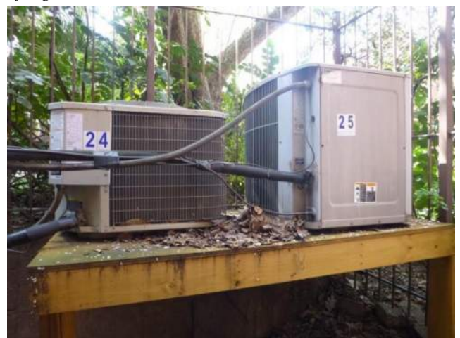
Figure 3.4-12. View of condensing units at the southwest corner of Egleston Hall.
