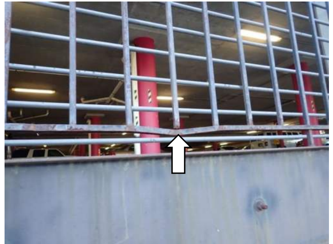
Figure 5.2-10. Failed fence element at parking garage opening.
