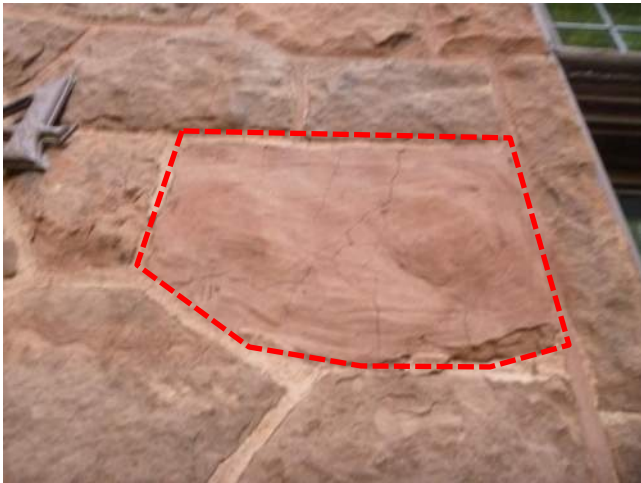
Figure 3.2-3. View of a failed patch repair in the stone masonry on the Egleston building.
