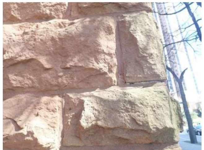
Figure 2.2-6. Hairline cracks and shallow surface delaminations in the brown sandstone facade.
