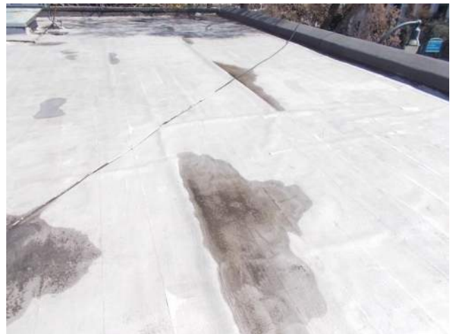
Figure 6.3-16. Small, localized areas of ponding water were observed on the roof.
