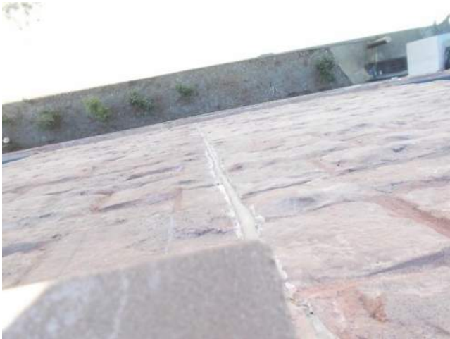
Figure 5.1-11. Expansion joint in the outer wall at the northwest corner of the roof does not continue up and over the wall to the roof.
