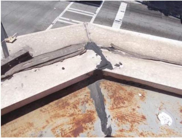
Figure 6.2C-17. The metal coping is corroded and the splice/lap joint seals are weathered, deteriorated, cracked and failed.
