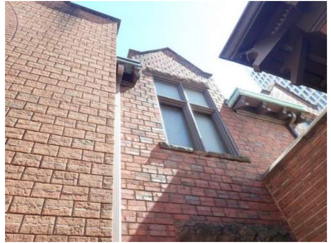
Figure 2.2-14. The brick masonry was weathered and mortar joints were eroded.
