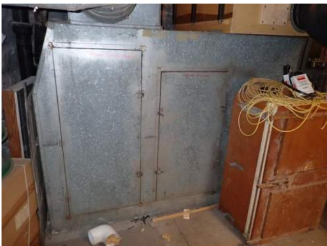
Figure 2.4-11. View of the organ blower for the Church and Chapel.
