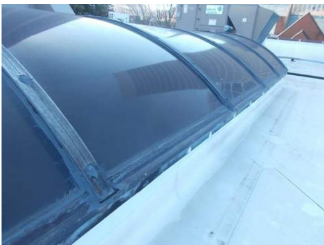
Figure 4.1-19. Sealant at skylight was chalky and generally deteriorated
