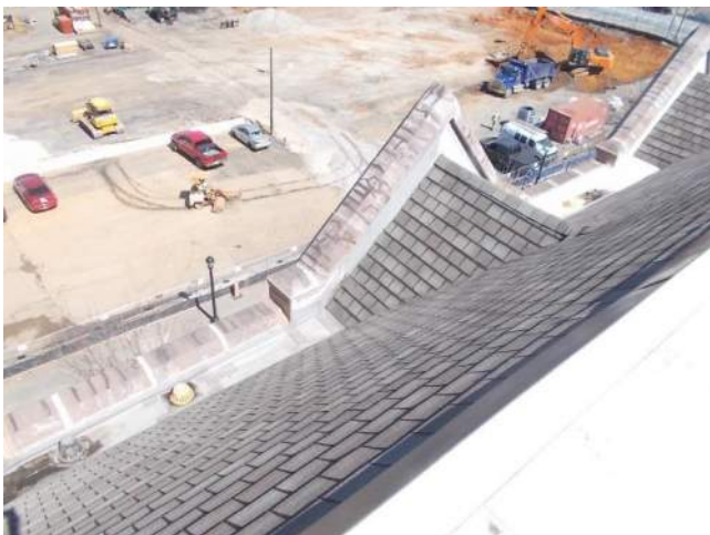
Figure 5.1-19. Cast stone coping with crazing cracks, many repaired with a liquid applied material.
