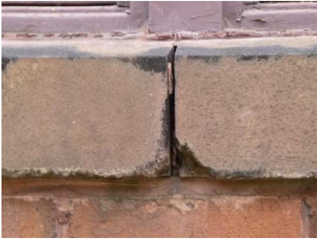
Figure 4.2-11. View of a minor spall and missing mortar at a cast stone window sill.
