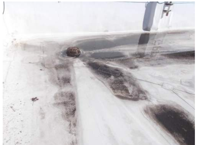
Figure 4.1-6. Ponding water around a roof area drain.
