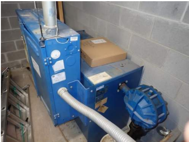
Figure 2.5-1. View of the elevator hydraulics and control system located in the mechanical/storage room.
