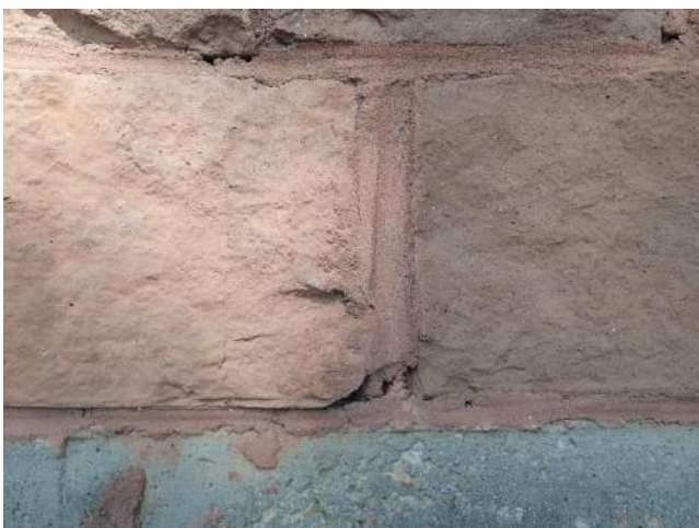
Figure 7.5-5. View of deteriorated mortar joints in the stone masonry of the storage shed.
