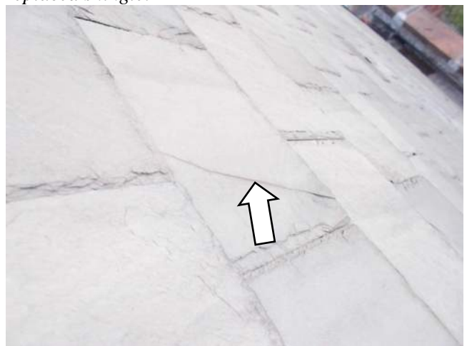
Figure 3.1-8. View of a crack in an isolated slate roofing tile.
