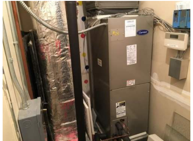
Figure 3.4-4. View of an air handling unit in a mechanical closet adjacent to the music staff offices.
