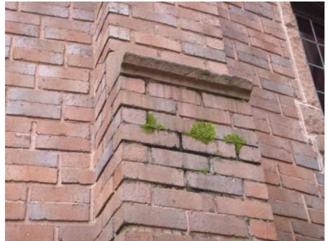
Figure 3.2-16. View of apparent organic growth on a buttress on the Egleston building.
