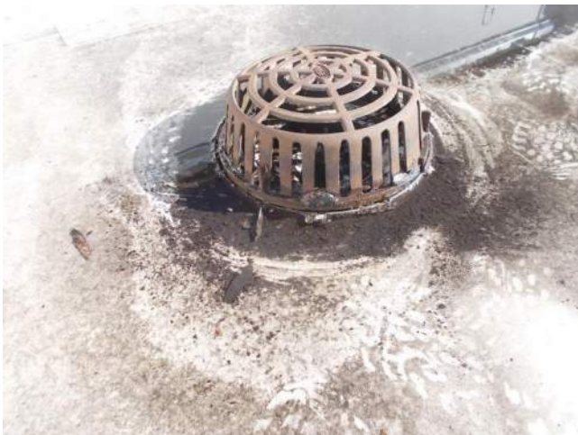
Figure 4.1-17. Weeps in the clamping rings clogged with organic debris.
