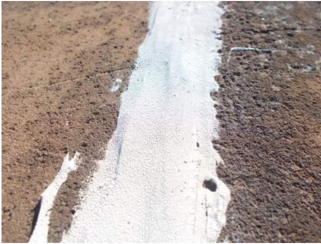
Figure 4.1-9. Deteriorated sealant between the coping joints.
