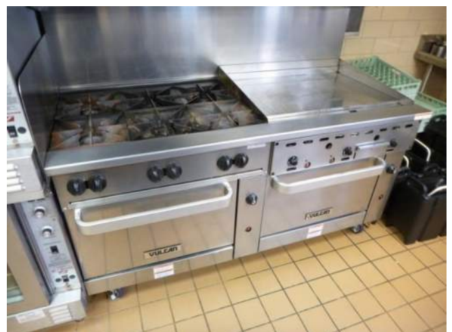
Figure 4.3-8. View of the stovetop and oven equipment in the Parish House kitchen.
