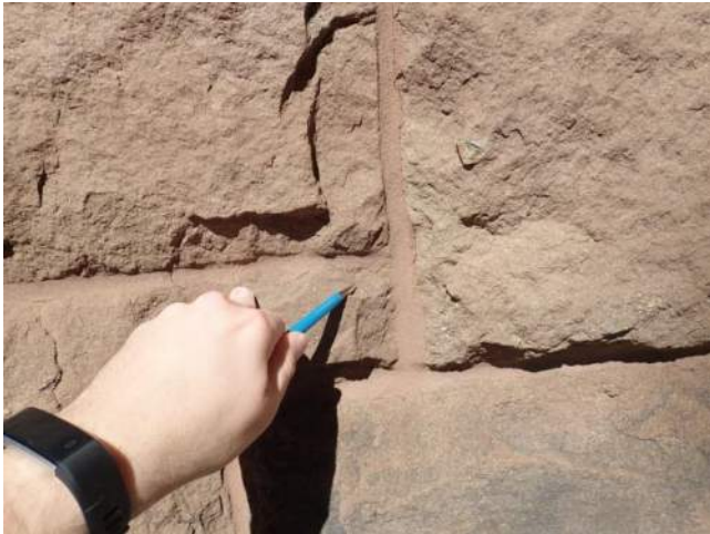
Figure 2.2-7. Hairline cracks and shallow surface delaminations in the brown sandstone facade.
