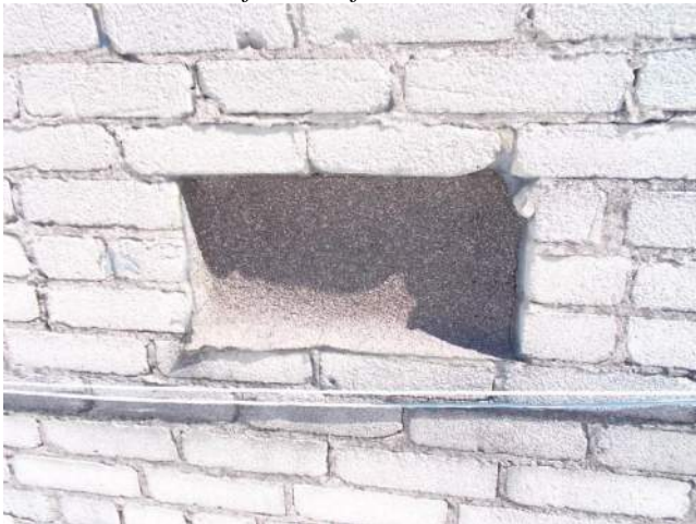
Figure 6.2C-13. Opening in the adjacent brick masonry wall covered with a granular surfaced modified bitumen membrane.
