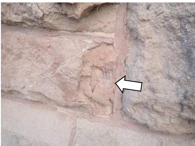
Figure 2.2-11. Exfoliation of a sandstone unit.
