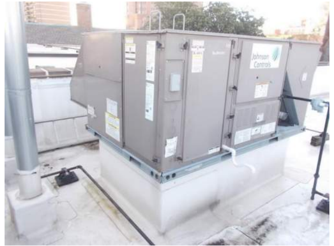
Figure 4.4-2. View of a RTU at the Parish House roof level.
