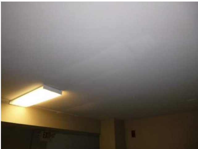
Figure 6.5-9. View of previous repairs to an area of ceiling on the second floor of Tate Hall.
