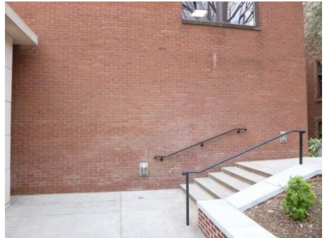
Figure 4.2-8. View of isolated areas of efflorescence on the south elevation.
