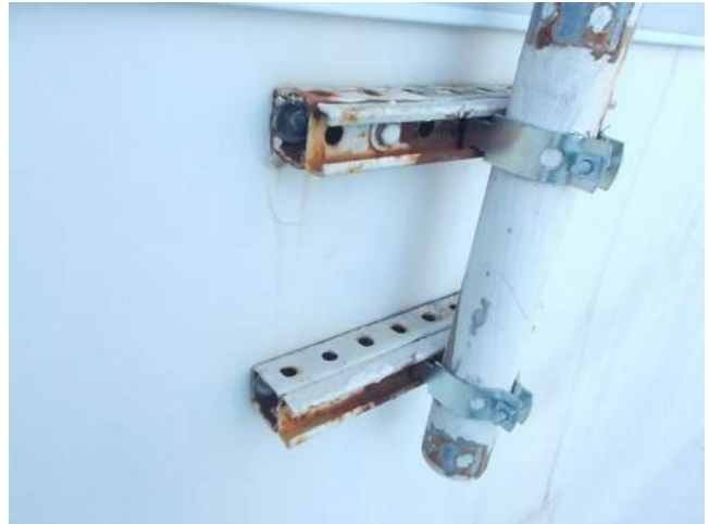
Figure 4.1-16. Unsealed bolt anchors securing the metal uni-strut that supports the lighting.
