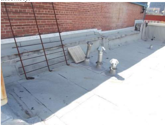
Figure 6.2A-11. Materials stored or resting directly on the roof membrane surface.
