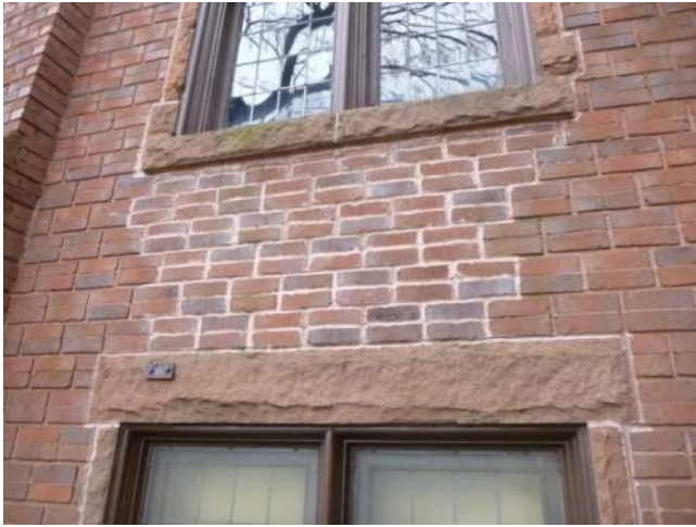
Figure 3.2-13. View of sealant repairs at an area of brick masonry on the south elevation.
