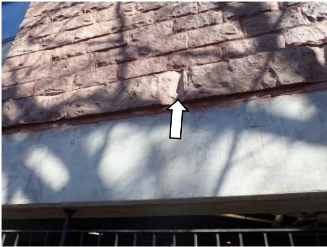
Figure 5.2-1. Isolated spalls at a manufactured stone masonry ledge.
