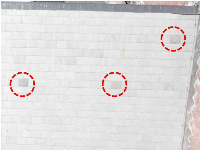
Figure 2.1-11. Slate roofing shingles appear to have been replaced as they are a different color.
