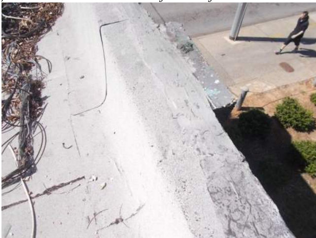
Figure 6.2A-5. Liquid membrane patches and apparent repair attempts on the terminations on the copings.
