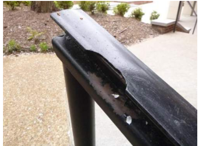
Figure 7.1-4. View of damaged guardrail at a courtyard site stair.
