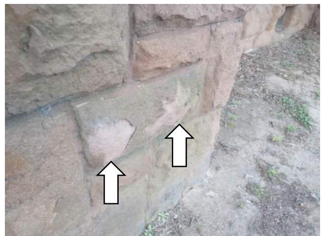
Figure 2.2-12. Exfoliation of a sandstone unit.
