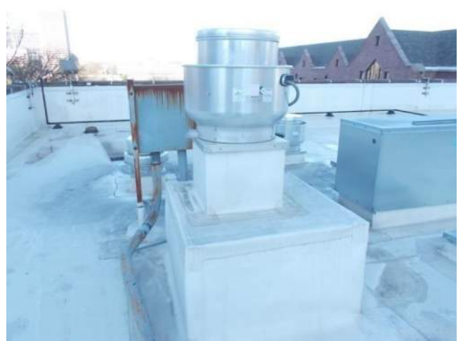
Figure 4.4-4. View of an exhaust fan on the Parish House roof.
