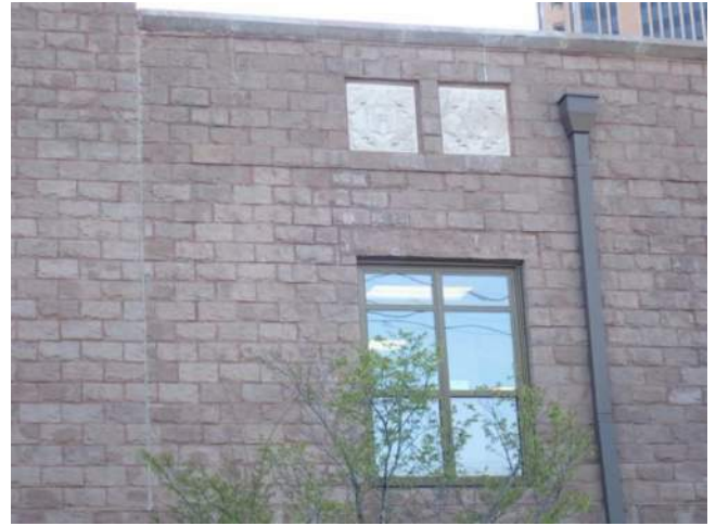
Figure 5.2-8. White haze on the face of the masonry.
