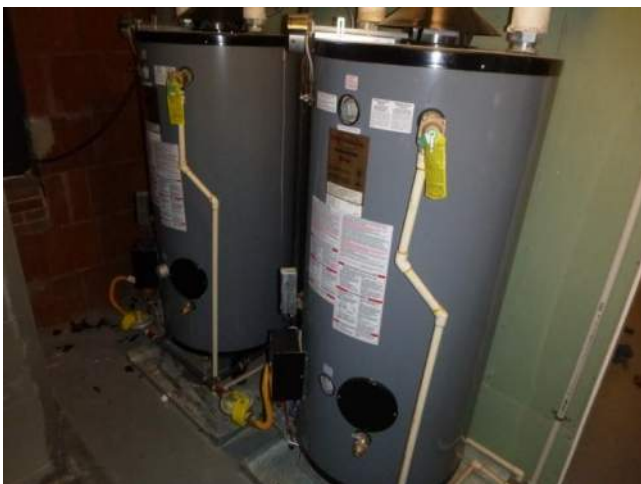
Figure 4.4-9. View of two 76 gallon hot water storage tanks in the mechanical room on the third floor.
