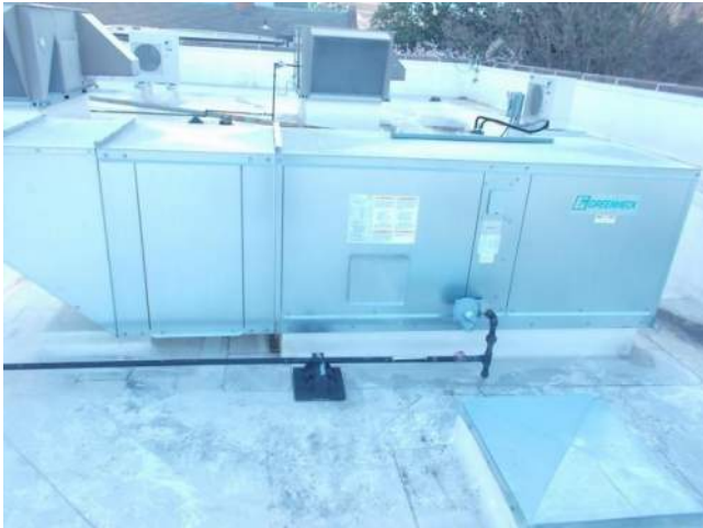
Figure 4.4-7. View of the makeup air unit on at the Parish House roof level.
