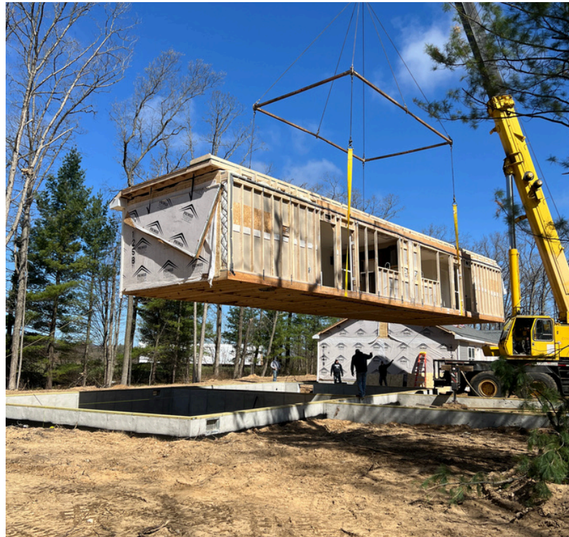
Duplex units in the City of Harrison, Clare County, that received funding from the MSHDA MI Neighborhood program are set on their foundation.
