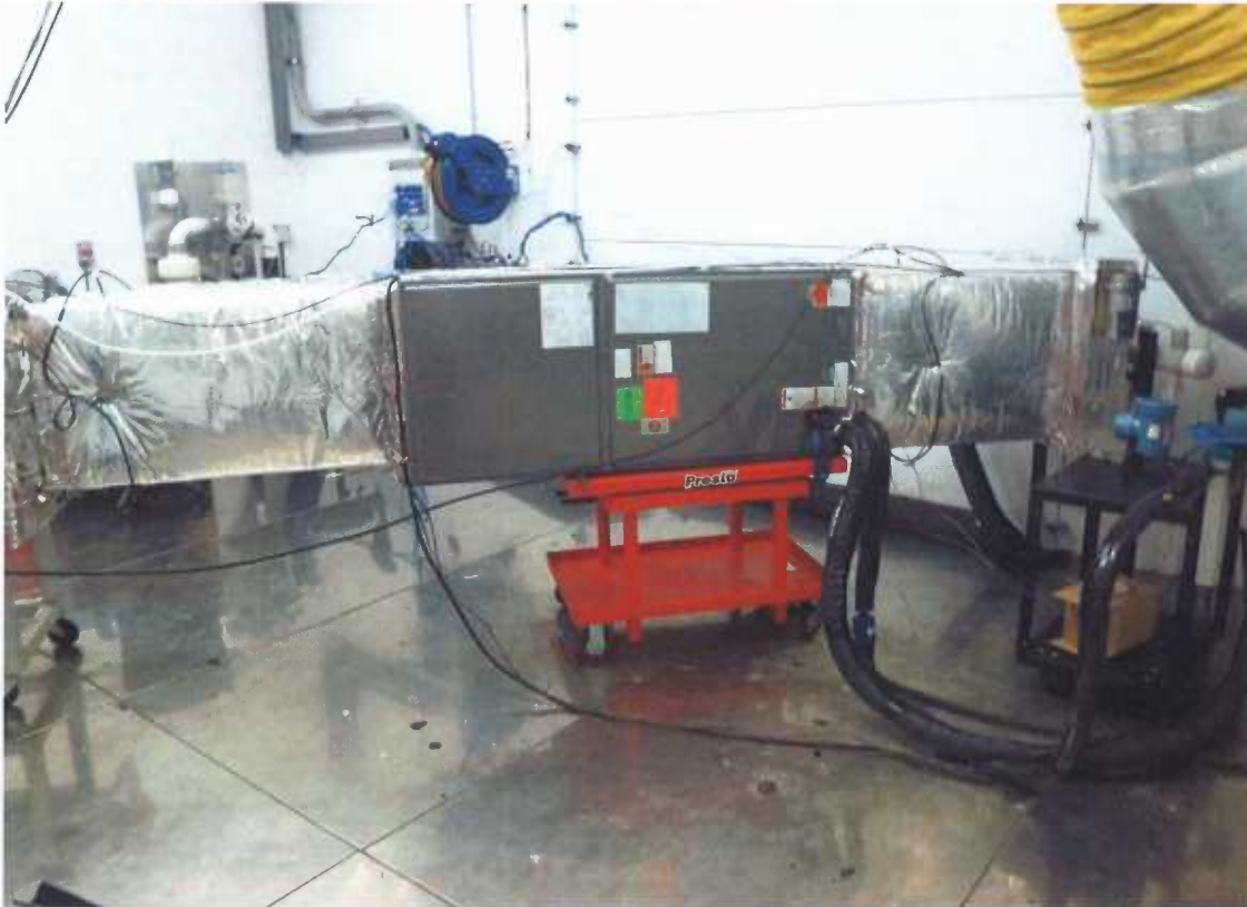
Photo 6 - Air Handler Setup
