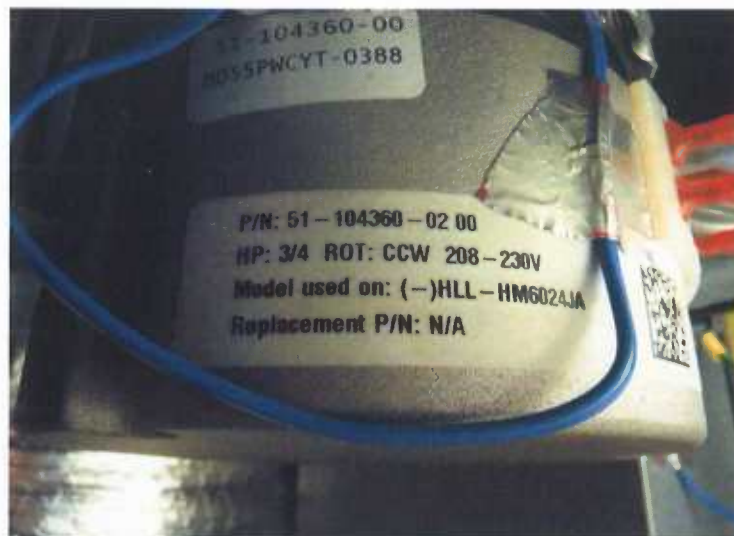
Photo 3 - Indoor Blower Motor Nameplate
